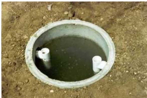
Figure B17.1: Grease interceptor
