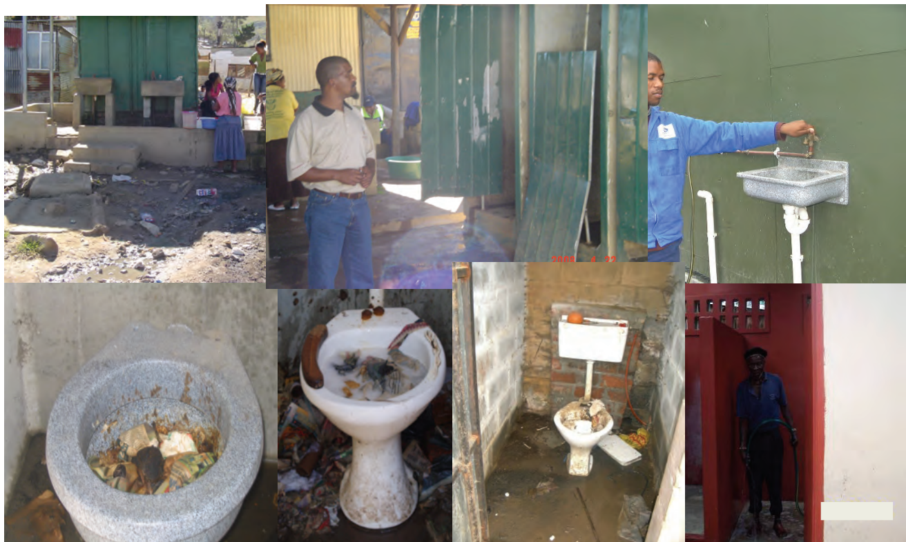
Figure 13: View of the O&M issues at the ablution facilities
