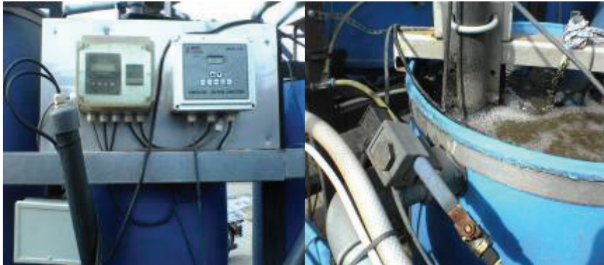
Photograph 11 DO concentration meter in last aerobic tank and solenoid valve
