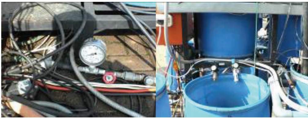
Photograph 15 Air inlet control and air water traps
