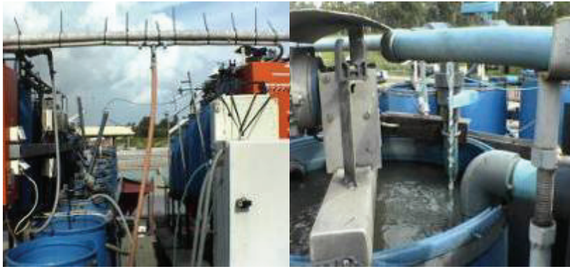
Photograph 7 Pilot plant supply and tank inlet
