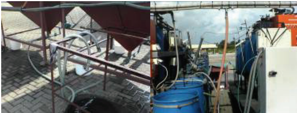
Photograph 13 Sludge waste points.
