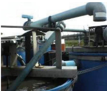
Photograph 8 The s-recycle inlet into tank 2
