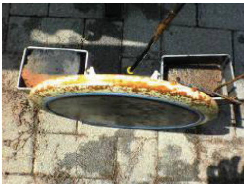
Photograph 16 Nopol disc with support frame and inlet pipe
