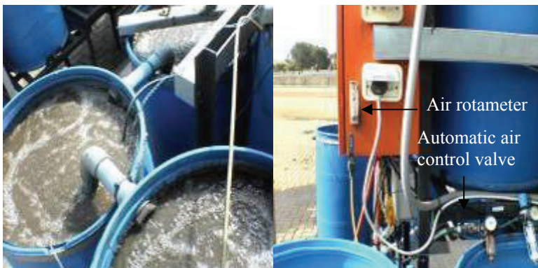
Photograph 10 First three aerobic tanks and air control valve
