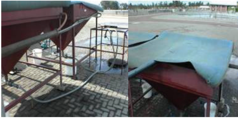
Photograph 12 Settling tank drain and covers to block out sunrays
