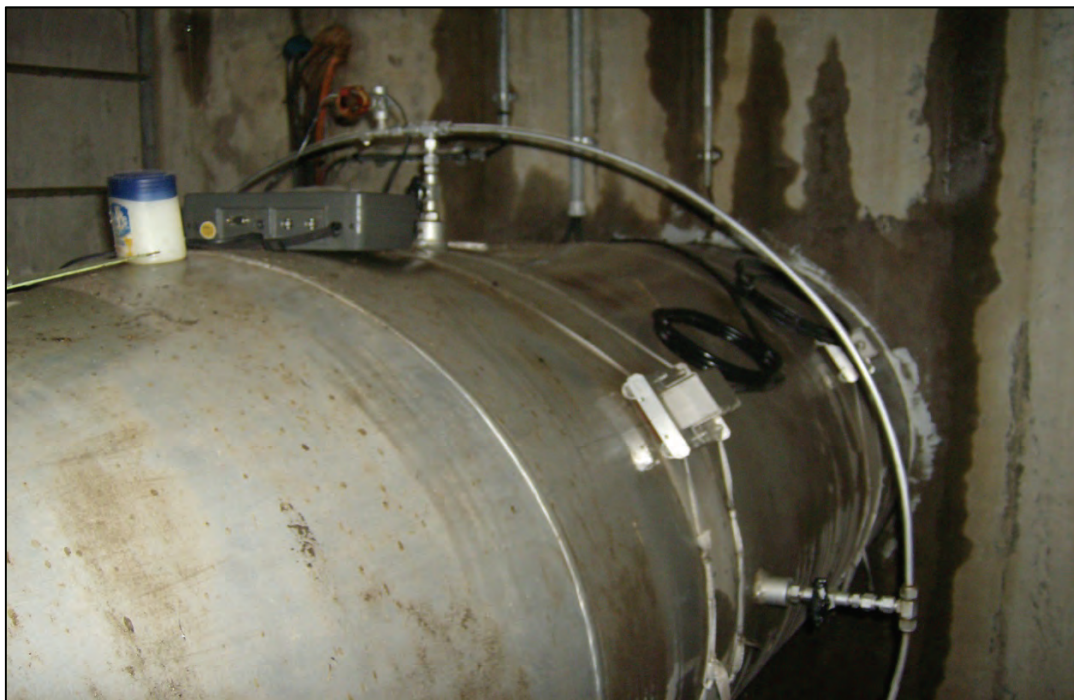
Figure 4-31: Fuji Portaflow flow meter
