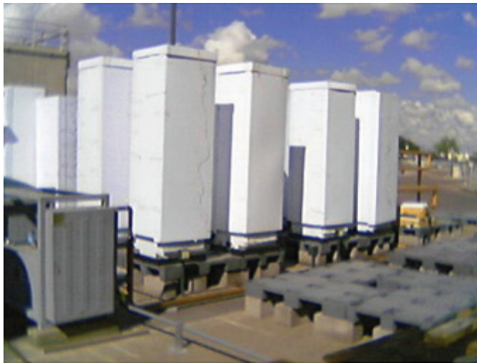
FIGURE 18. 20 m 3 /d RO CONCENTRATE TREATMENT PLANT BUILT BY L'EAU (L'EAU, 2006)
