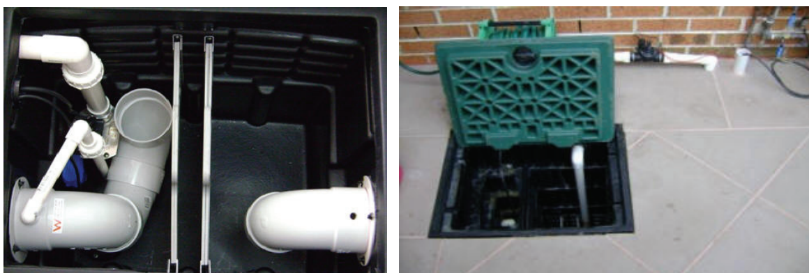
Figure 66 Example of a SmartPit system from Wattworks (from http://www.wattworks.com.au ).
