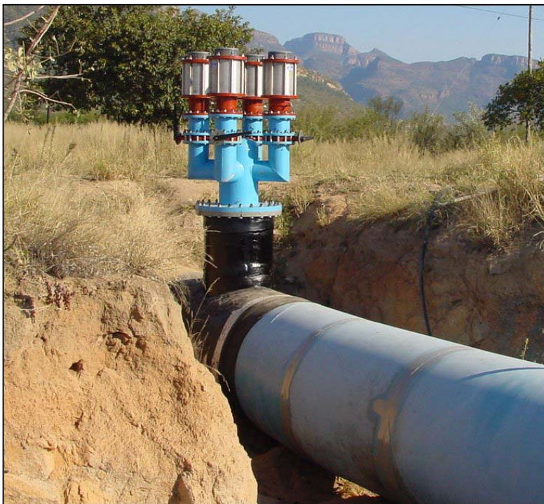
Figure 8.5: Four air valves on a manifold (above ground installation)
