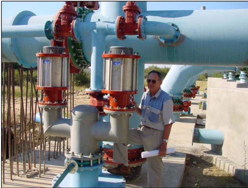
Figures 8.4: Two air valves on a manifold (above ground installation)
