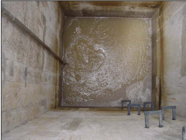
Figure 3.5: A photo of white water in surge tower (Buffalo River abstraction, East London, South Africa)
