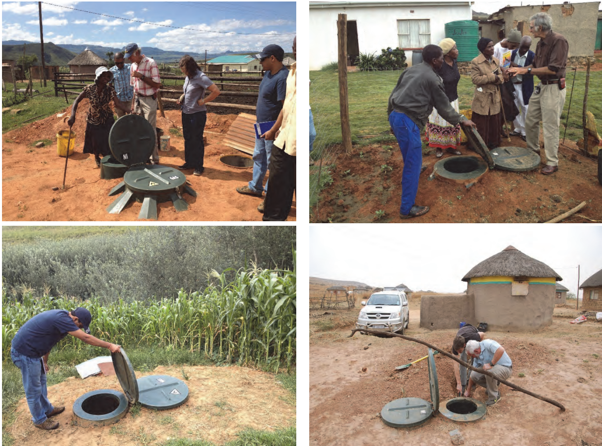
Plate 4.3: Completed installation - clockwise from top left; Obonjaneni pilot site, New Stand pilot site, Potshini pilot site, Okhombe pilot site, in KZN.
