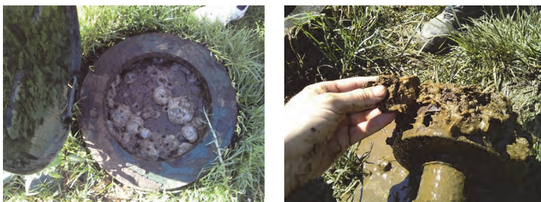
Plate 9.2: Blocked digester, requiring emptying and re-commissioning.
