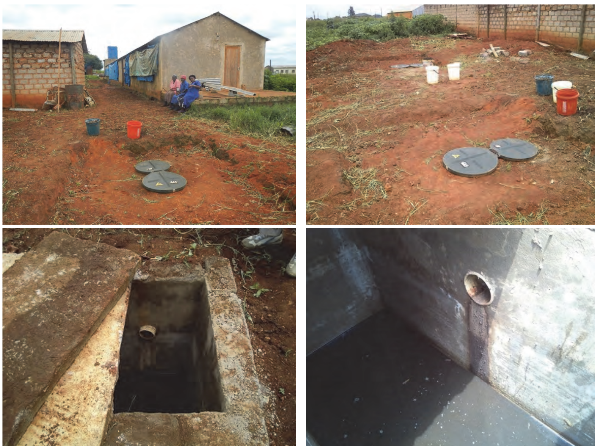
Plate 4.8: Biodigesters installed at Maila crèche.
