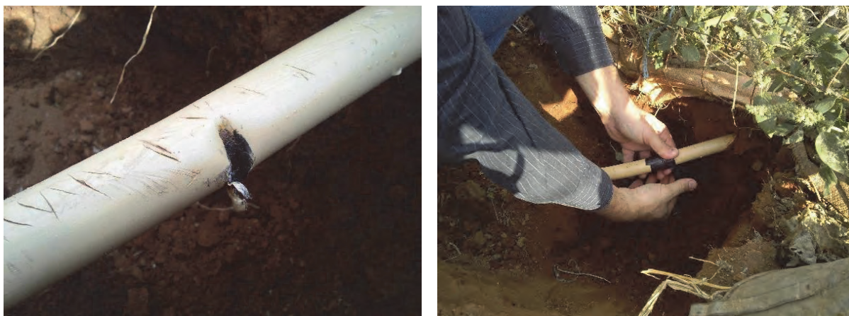
Plate 9.1: Minor repair required after household damaged a subsurface gas line with a new fence post.
