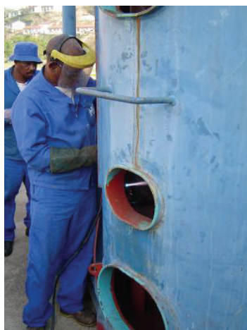
The Operational Information tool records any maintenance that is carried out on Drinking Water Treatment infrastructure.
