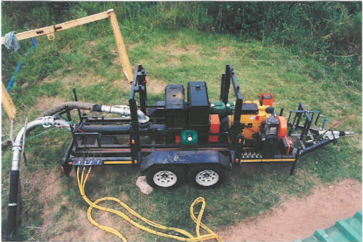
Figure 6.4 : Mobile trailer mounted test unit in operation (pipes unloaded and motive pump running)
