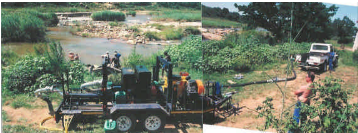
Figure 7.1 : Test pilot plant in operation at the Sabie River Intake (Refer also to Figure 5.4 which shows the intake viewed from the river side).
