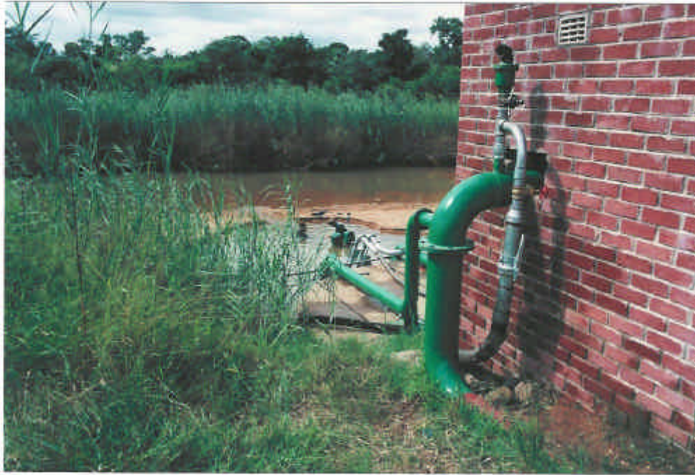
Figure 6.6 : The tap-off of the fixed pump's motive pipe from the raw water discharge pipe at the Sand River intake pumphouse. (Sandbank in river visible in background).
