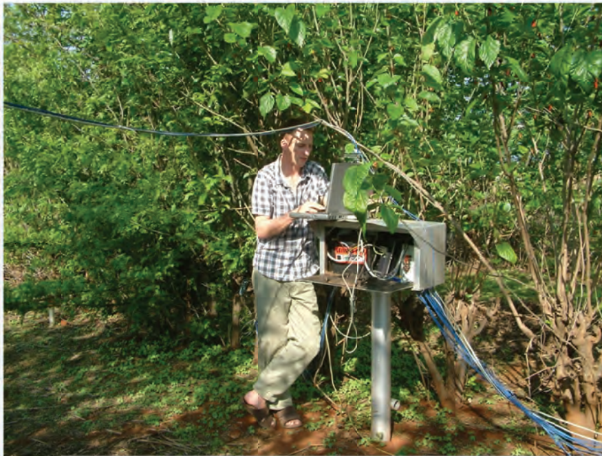
Plate 8.5 Down loading data from the HPV installation at the Mahlobo agroforestry site. The RR1 battery, CR 1000 data logger, Campbell AM 32A multiplexer and HPV relay control module can be seen in the security box.
