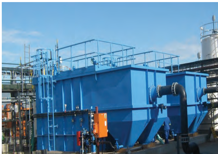
Figure 2-8: High rate clarifiers at the Tubatse site
