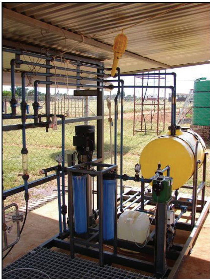
Figure 3.3 A picture of the cross-flow module reactor pilot water treatment plant
