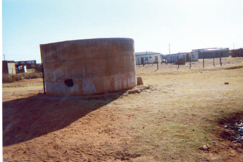
Picture 2. A non-functioning water service
