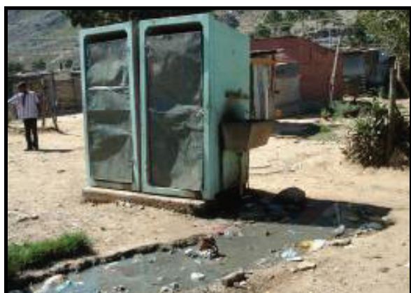
Collapsed toilet and leaking tapstand/ basin. Foul water is discharged down slope.
