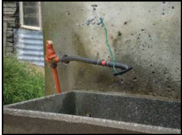
Home-grown modification. Wire crimp tap looks ugly although it works with minimal leakage.
