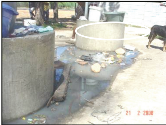
Figure 5.26: Poor drainage at the washing facilities in Simondium
