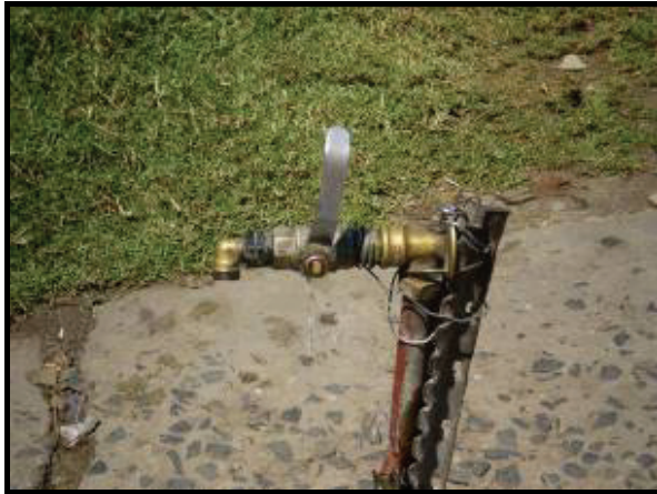
Secured tapstand at correct height for 25 litre bucket. Concrete base is secure and well drained.
