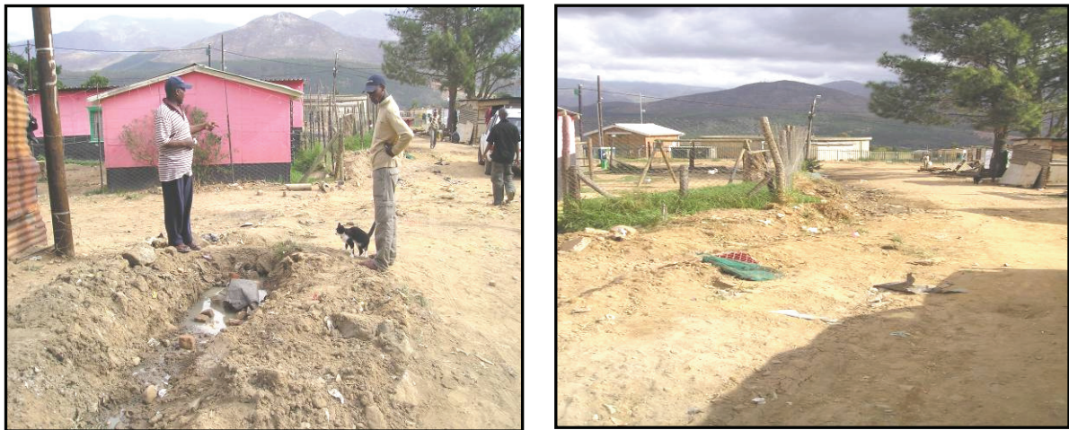
Figure 5.9: Problems with greywater initiatives at Langrug. Self-installed drainage pipe across road with the inlet blocked by rubble pushed there by a municipal grader (left). Note broken pipes in background. Crate grid broken by municipal grader (right)
