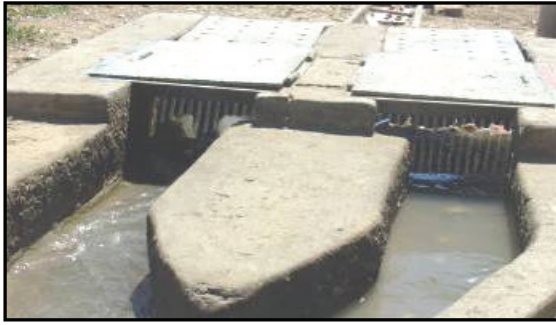
Figure 5.22: Structure diverting greywater to sewer in Fairyland
