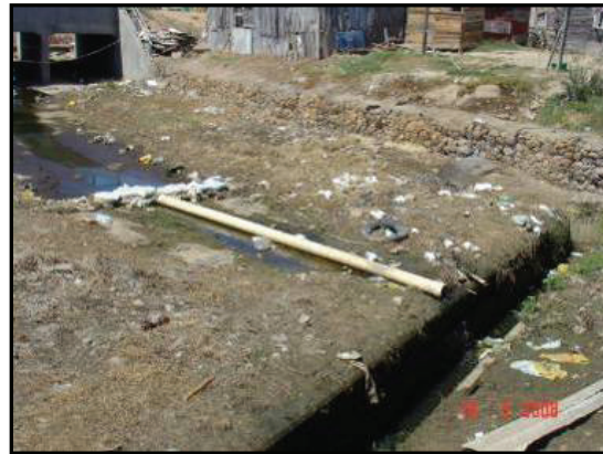
Figure 5.16: Stormwater diversion pipe in Drommedaris
