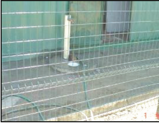
Figure 5.24: Standpipe draining to a channel outside an AACT unit in Fairyland
