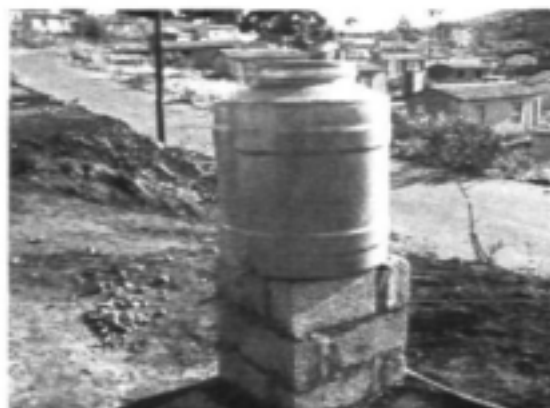
Figure D3.10: Mandela Park: controlled water supply
