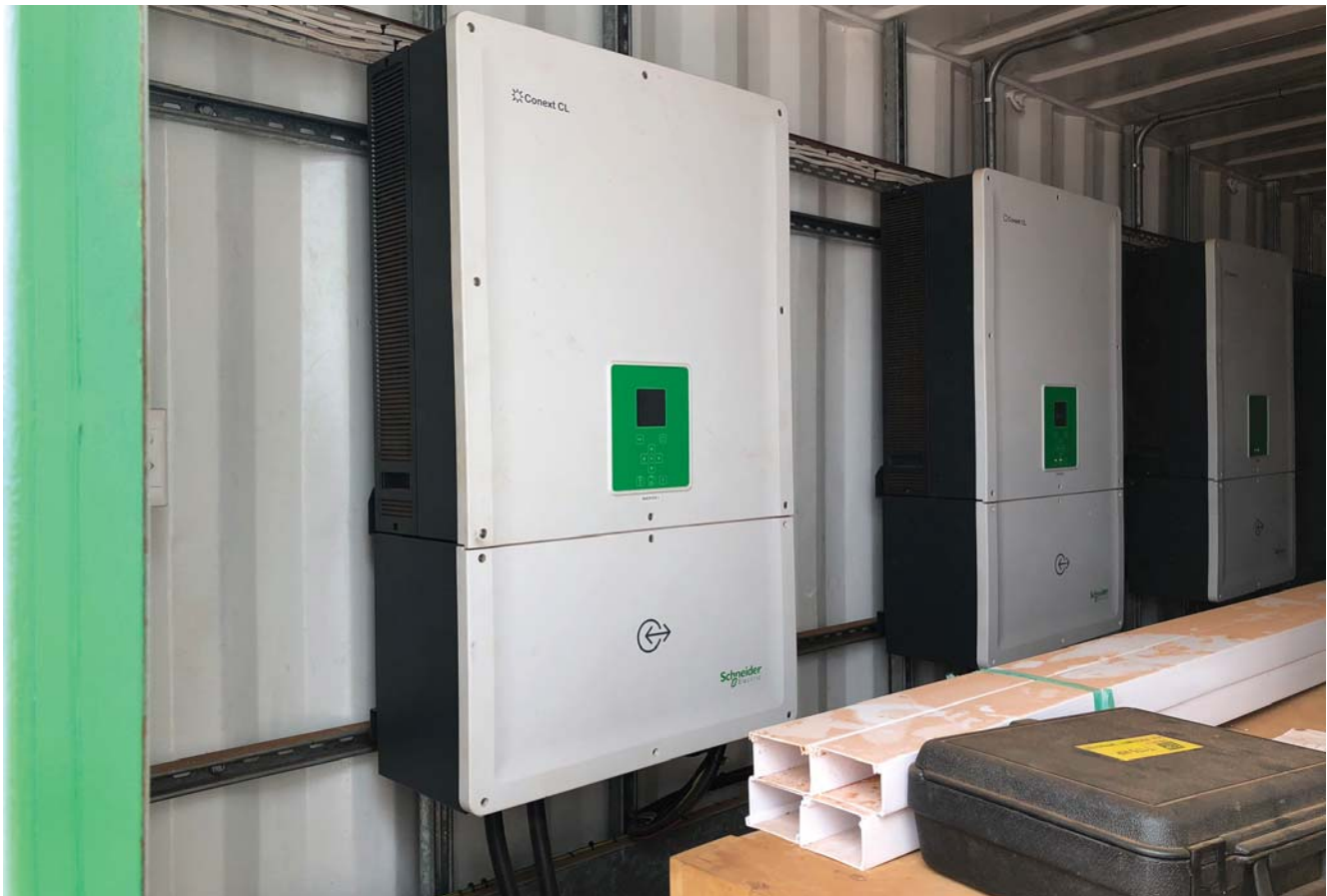
Becker Farm in Limpopo has a 250kWp DC system and 200kVA AC.
