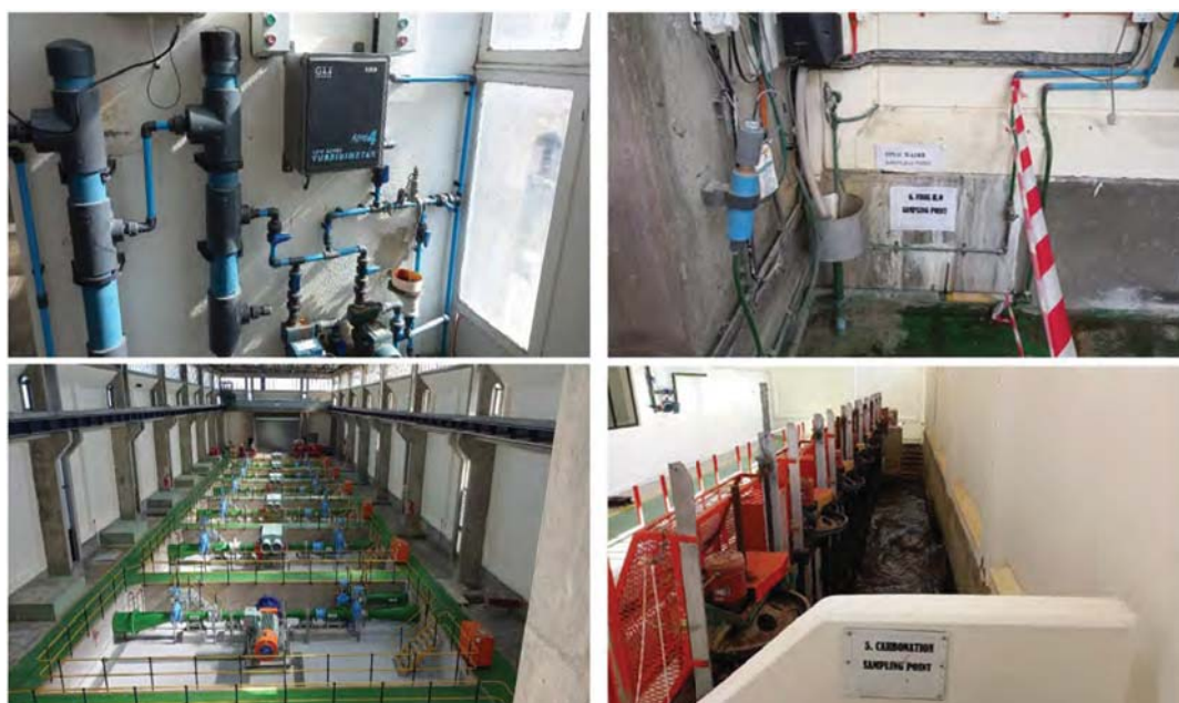
Figure 3-1: Drinking Water Treatment Plant sampling points.
