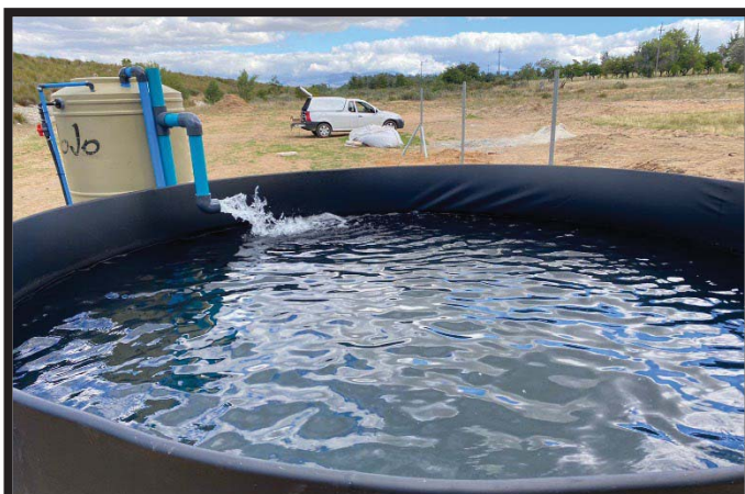
Figure 2.3.6 Water flowing in HP system
