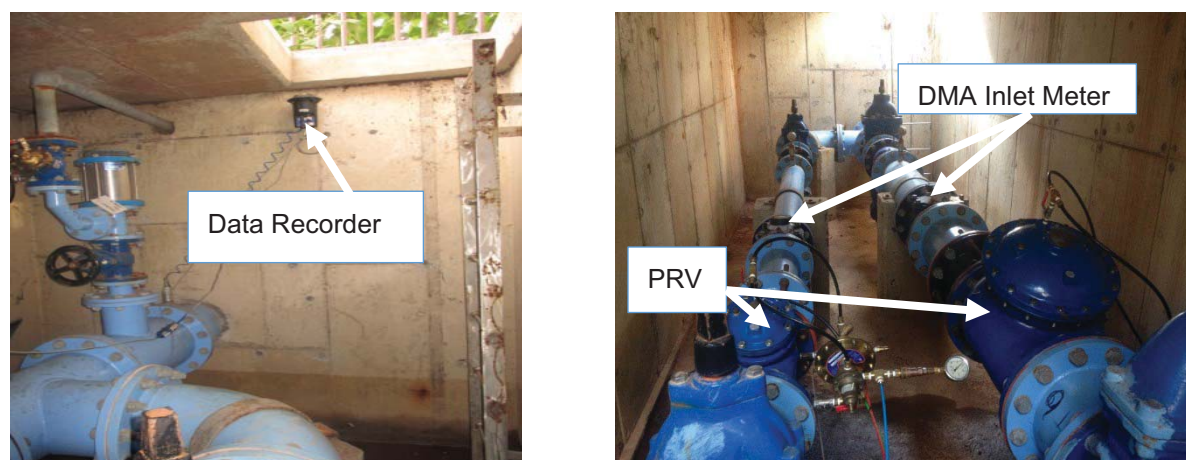
Figure 1: Typical data recorder installation at PRV
