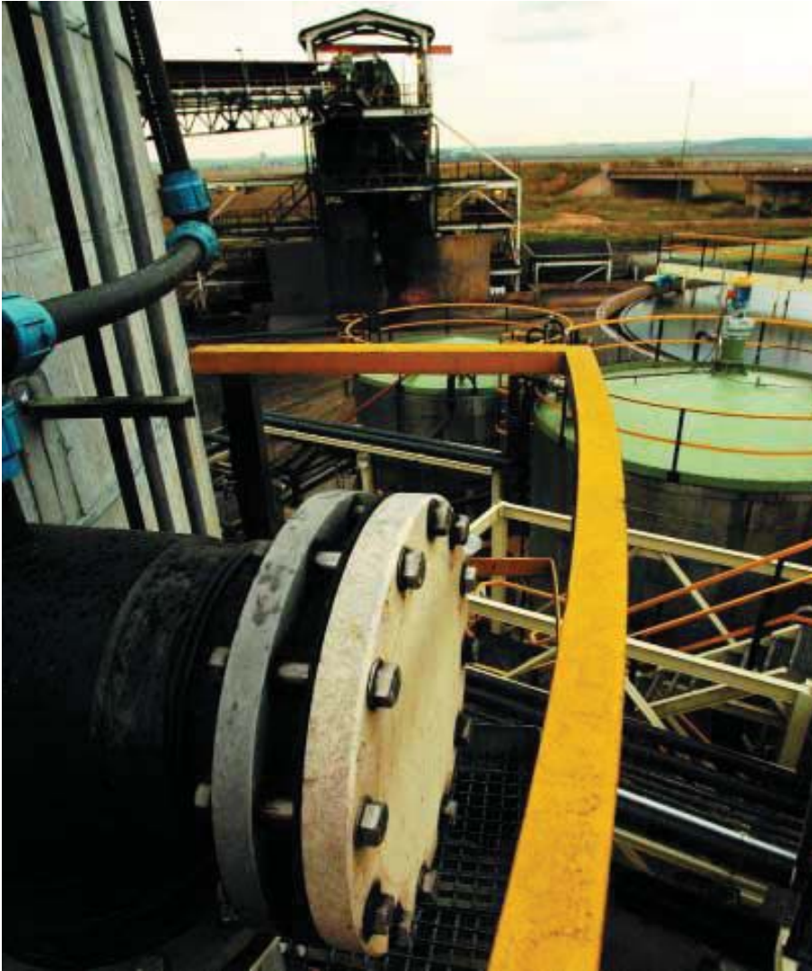
Figure 29: Biological water treatment plant at Landau Colliery
