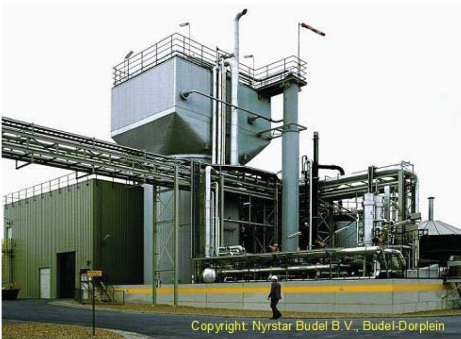
Figure 28: Full-scale biological sulphate reduction installation with hydrogen gas as electron donor
