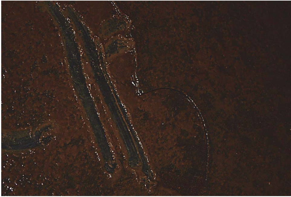
Figure 4-5: Biofilm growth on bitumen liner (Option 2B)
