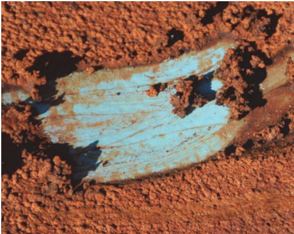
Figure 4-2 : Example of biofilm growth (Inyaka Pumping Main) in the raw water pipeline supplying the Bushbuckridge Water Treatment Plant
