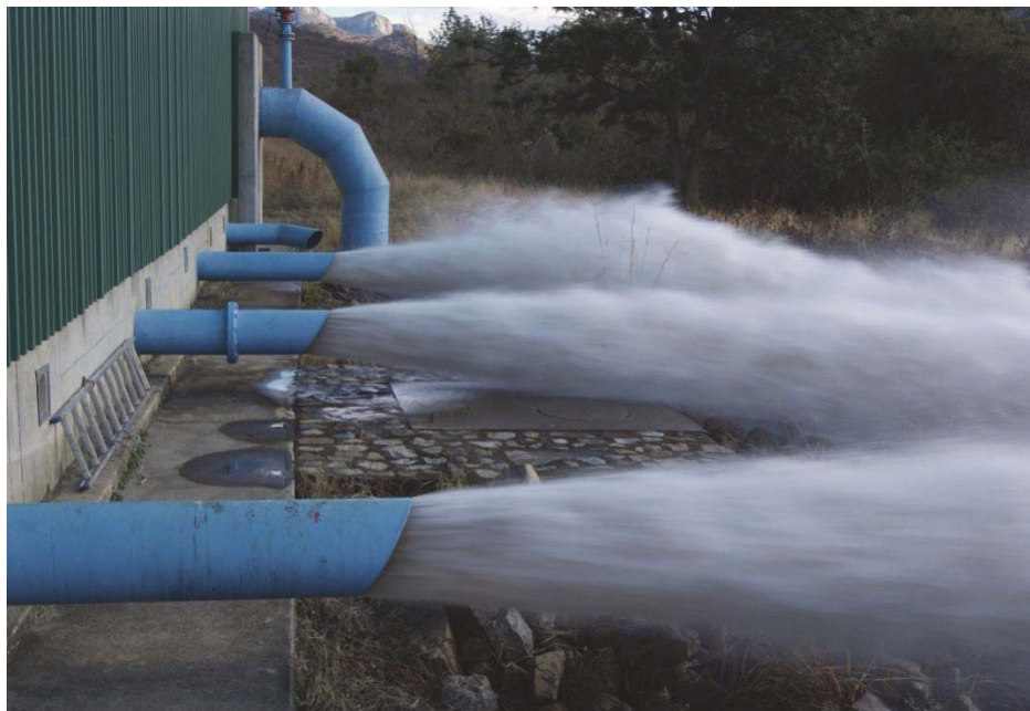
Figure 2-11: Three scour valves opened during the field test on the LBIS (July 2010)
