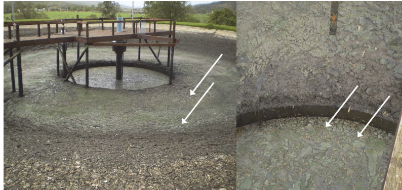
Figure 7 Evidence for sludge accumulation in the IPD (arrows; right panel) and the AFP (arrows; left panel) following drainage of water from the AFP.
