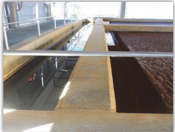
1 of 4 DAF tanks showing clear well channel
