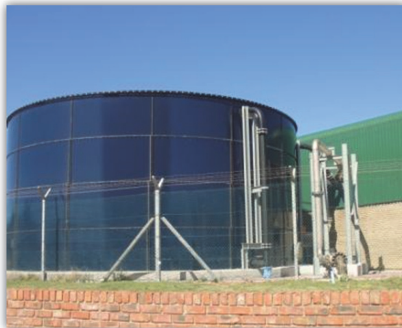
Backwash water storage tank
