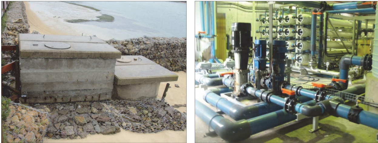
Figure 2.10: Albany Coast SWRO plant
