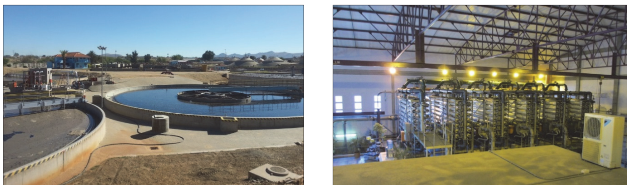
Figure 3.10: Gammams WWTP (left) and New Goreangab water reclamation plant (right)
