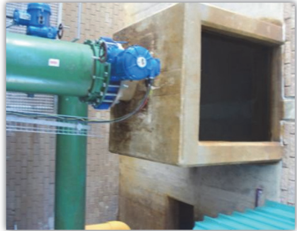
Pipe to sand-filters
