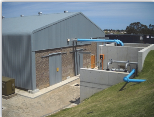
Backwash Recovery Tank and Pump Station
