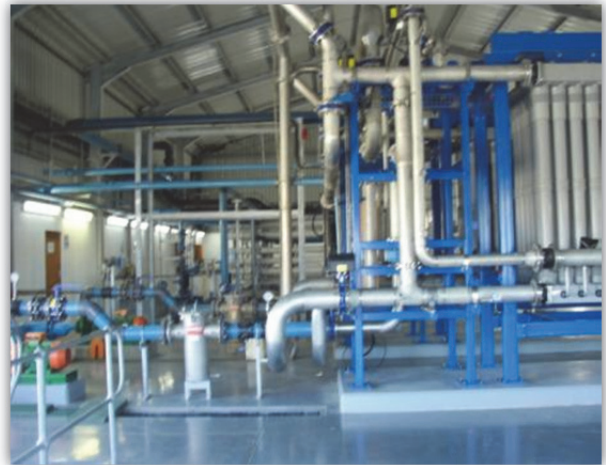
Automated backwash pumps
