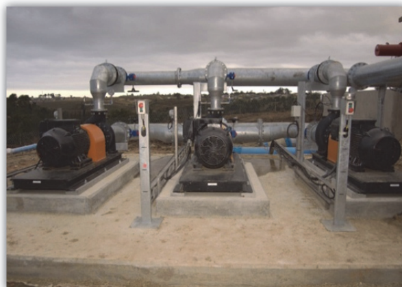
Filtrated Water Feed Pump Station (3 Pumps, 2 on duty and 1 on standby)
