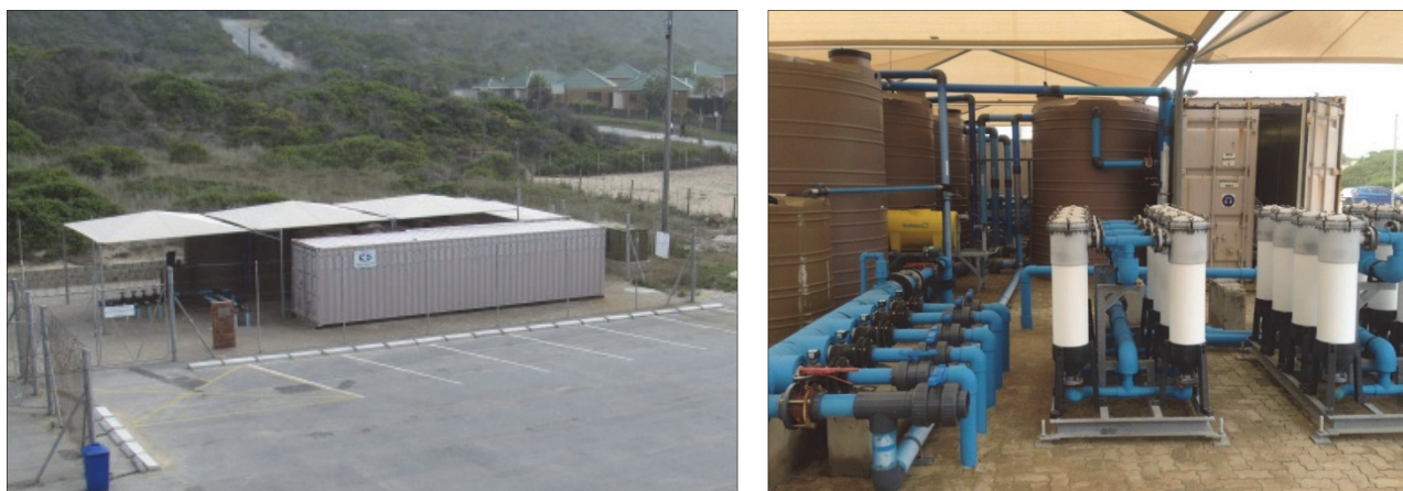
Figure 2.6: Sedgefield SWRO plant
