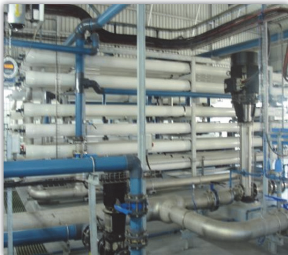
1 st stage RO unit
