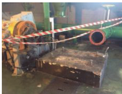
Plate B) Missing pump
