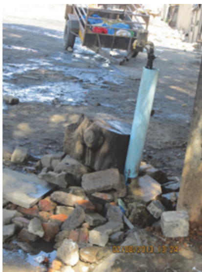
Figure 37 Municipal water saving device used to reduce wastage at a communal tap, Alexandria
