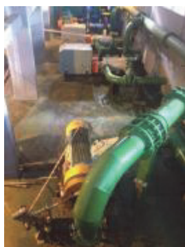
Plate A) Dysfunctional Pumps
