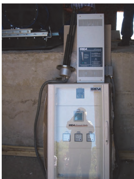
Figure 10-23: Control panel and regulator
