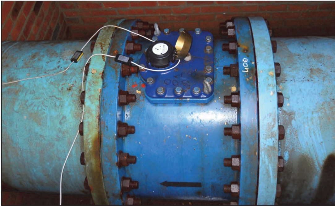
Figure 8-7: Flow measurement at Garsfontein Reservoir
