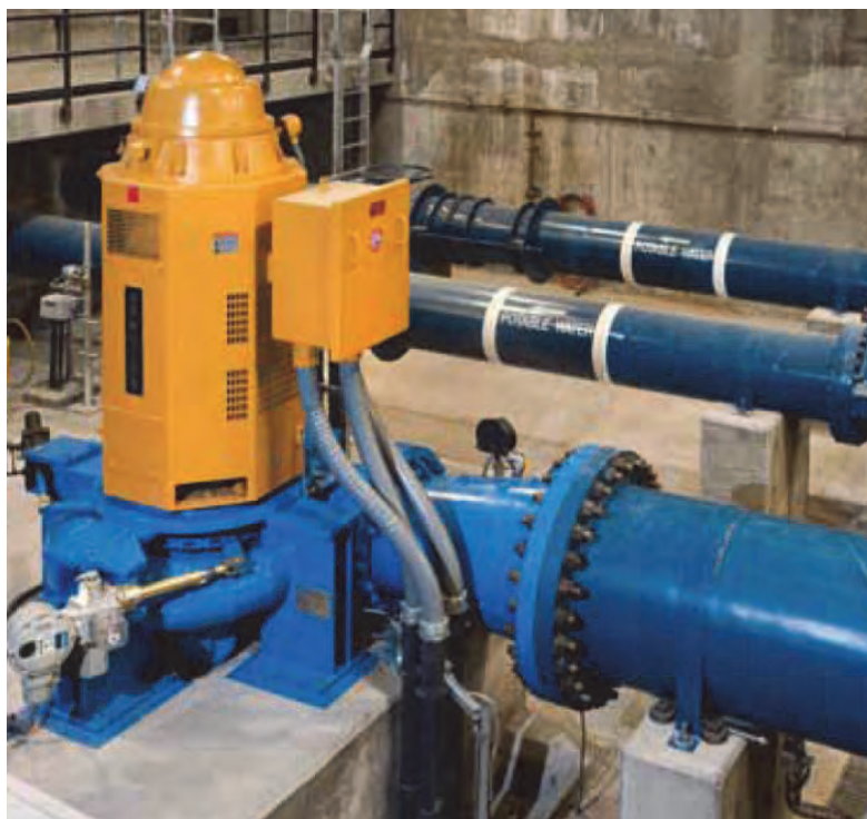
Figure 2-33: Hydroelectric turbine at Sloan Rate of Flow Control Station (SNWA, 2010)
