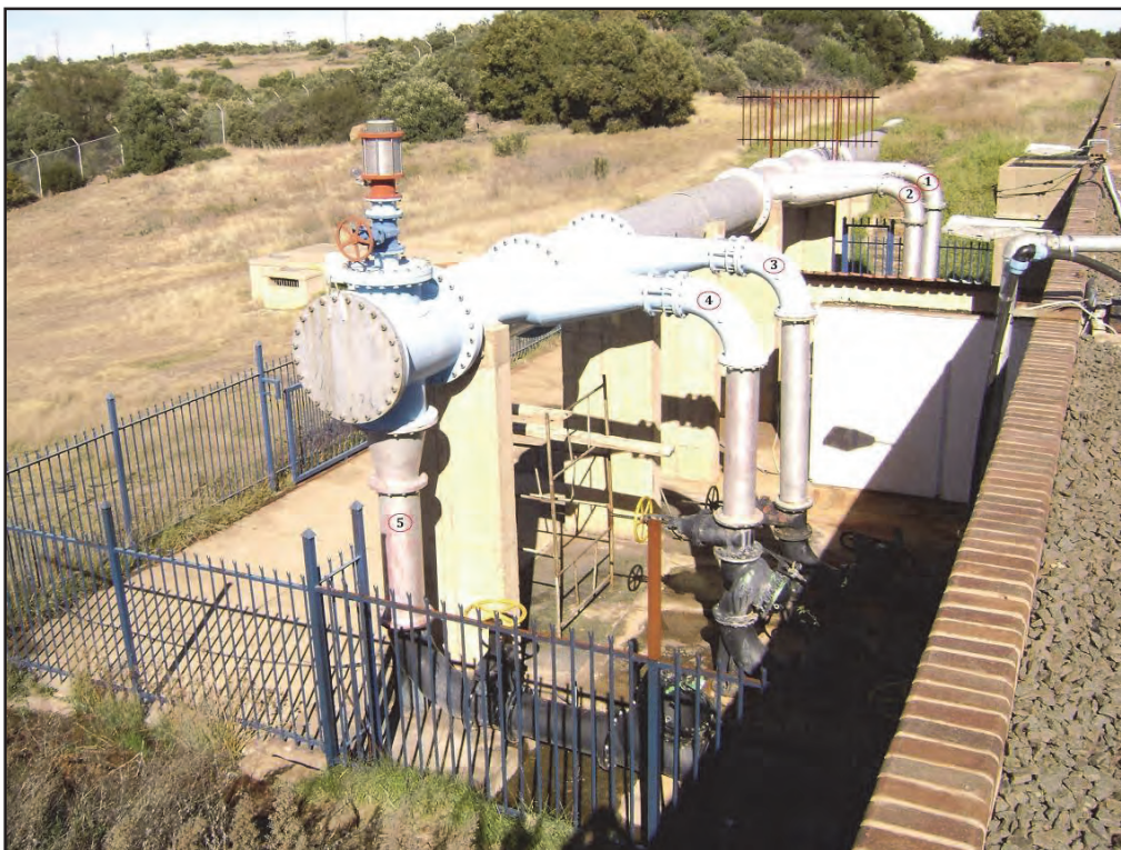
Figure 9-8: Control valves on the 5 branch pipes leading into Brandkop Reservoir
