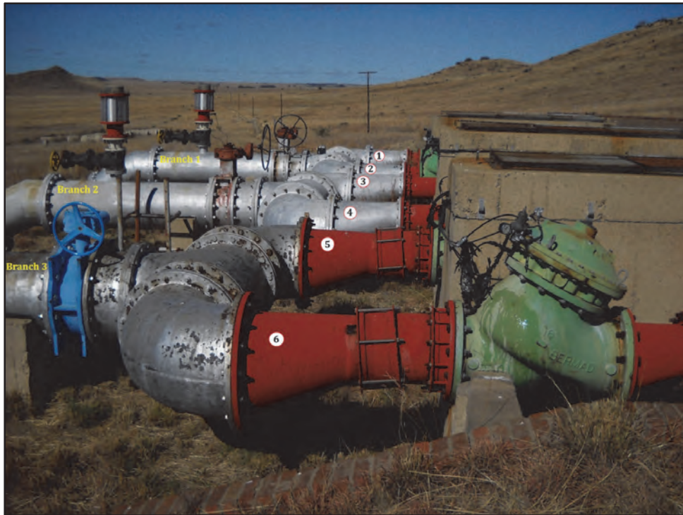
Figure 9-7: The six control valves on the 3 branches feeding into the Uitkijk Reservoir
