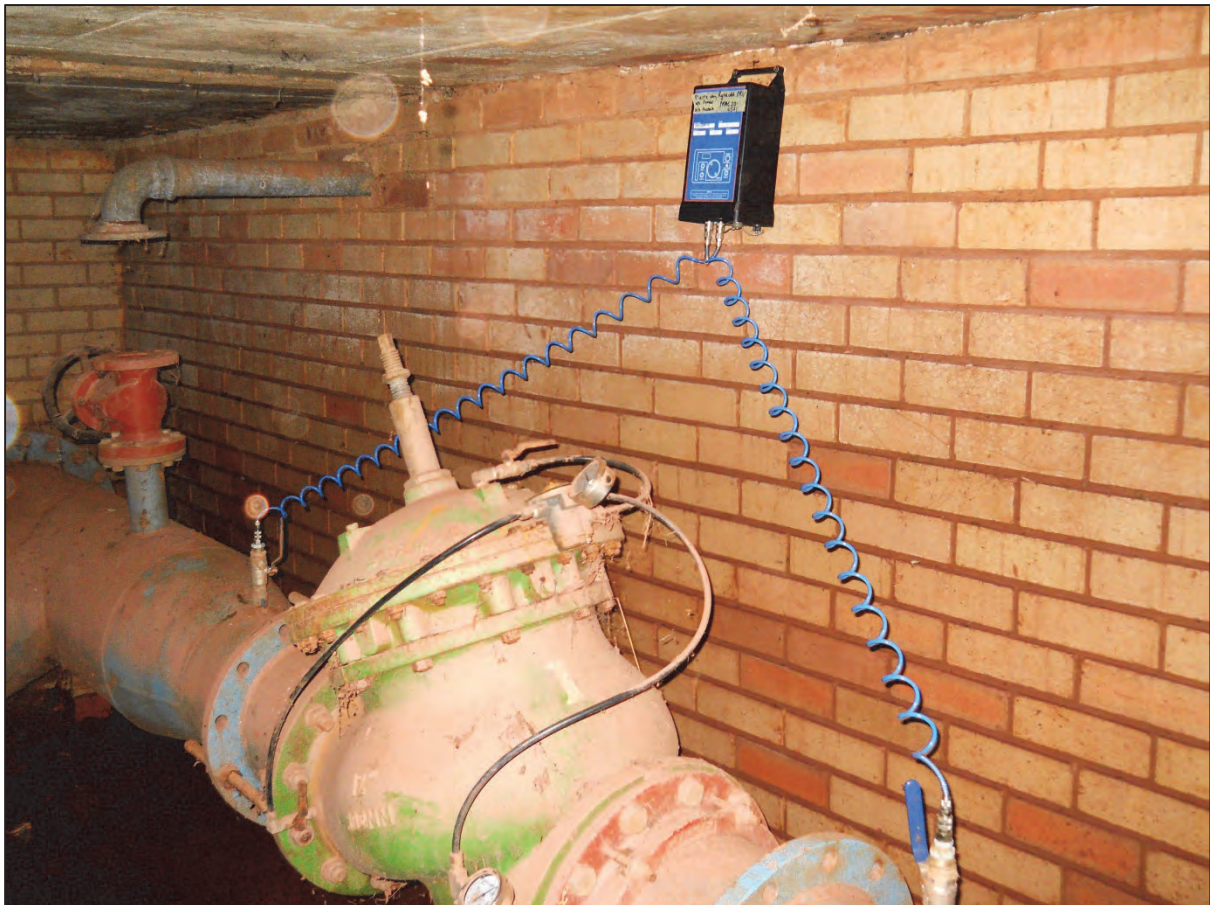
Figure 8-22: Pressure measurement at Pierre van Ryneveld pressure-reducing station
