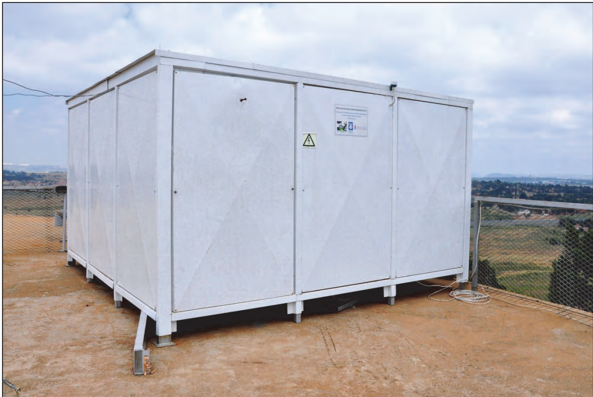
Figure 8-37: Pierre van Ryneveld turbine enclosure
