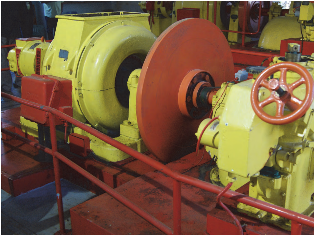
Figure 2-25: Flywheel (Ceres hydro power plant)
