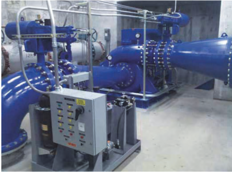
Figure 2-26: The City of Logan, Utah installed a Francis turbine to replace a pressure reducing valve (White, 2011)
