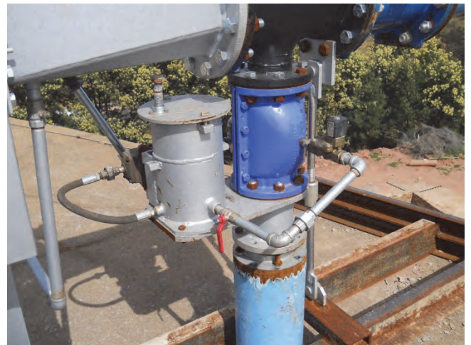
Figure 10-10: Emergency pinch valve (discharging into reservoir)
