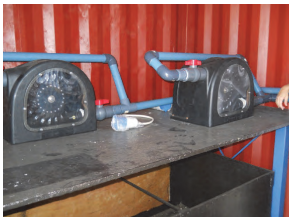
Figure 10-32: Two Powerspout pelton turbines
