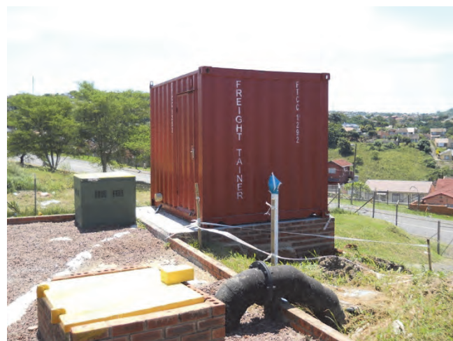
Figure 10-31: Turbine room (steel container) and connection point
