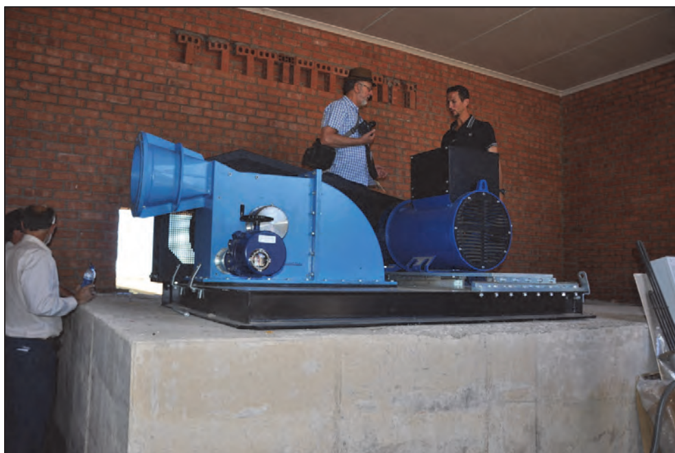
Figure vii: Brandkop hydropower installation
