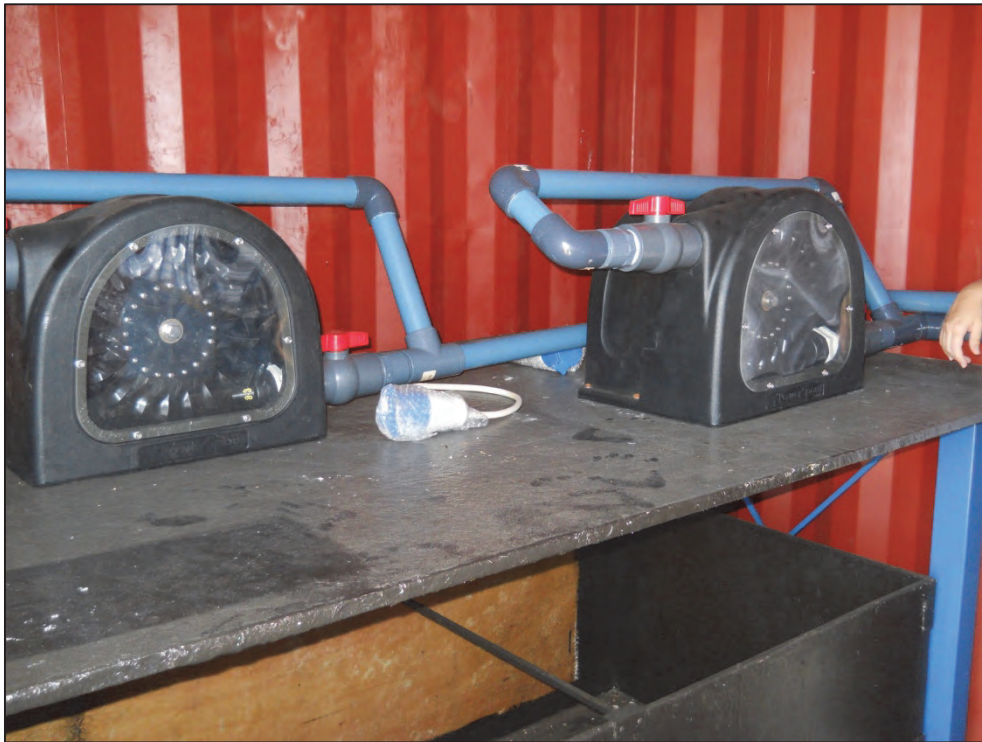
Figure viii: Newlands 2 Reservoir hydropower installation
