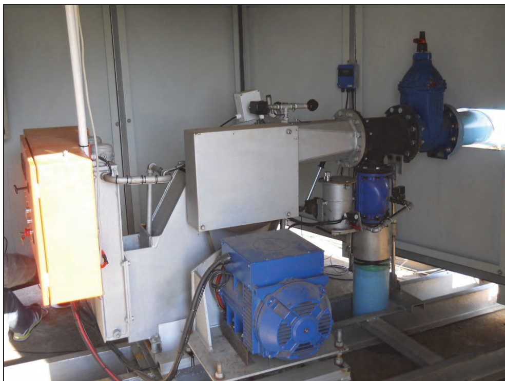
Figure vi: Pierre van Ryneveld hydropower installation
