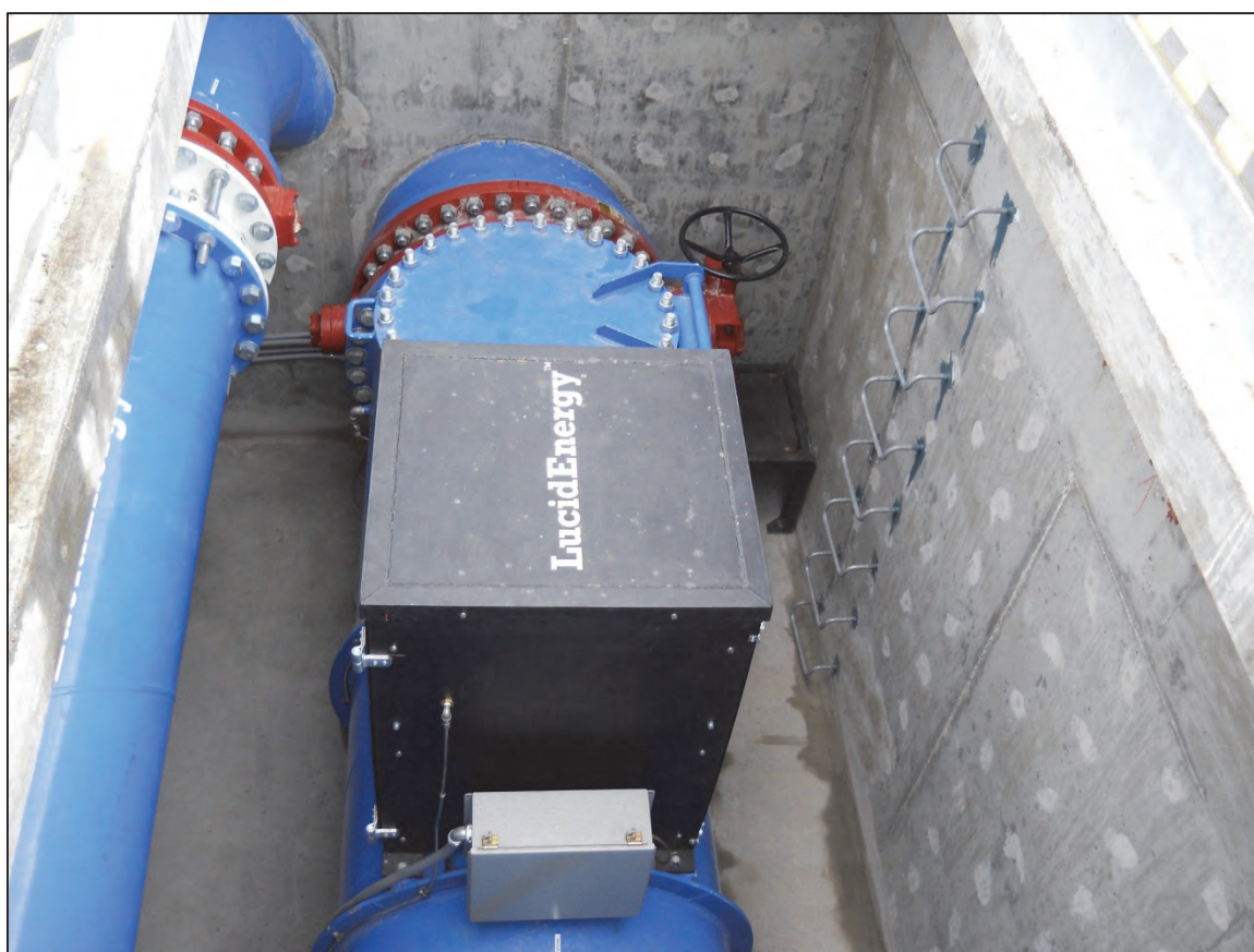
Figure 2-32: Installed LucidEnergy spherical turbine (Riverside, California)
