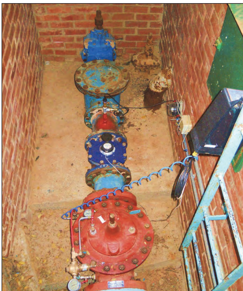
Figure 8-45: Pressure and flow measurement at Waterkloof Reservoir pressure-reducing station
