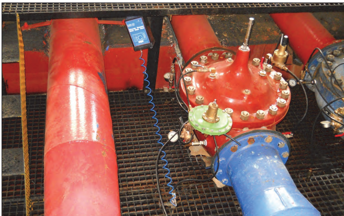
Figure 8-6: Pressure measurement at Garsfontein pressure-reducing station
