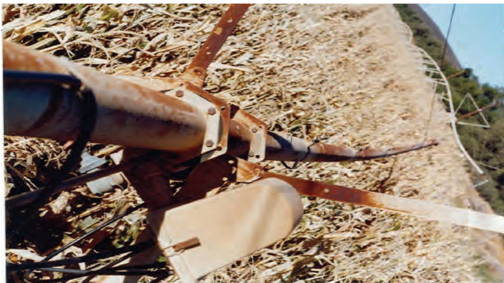
Figure 1. Effect of corrosion on irrigation system
