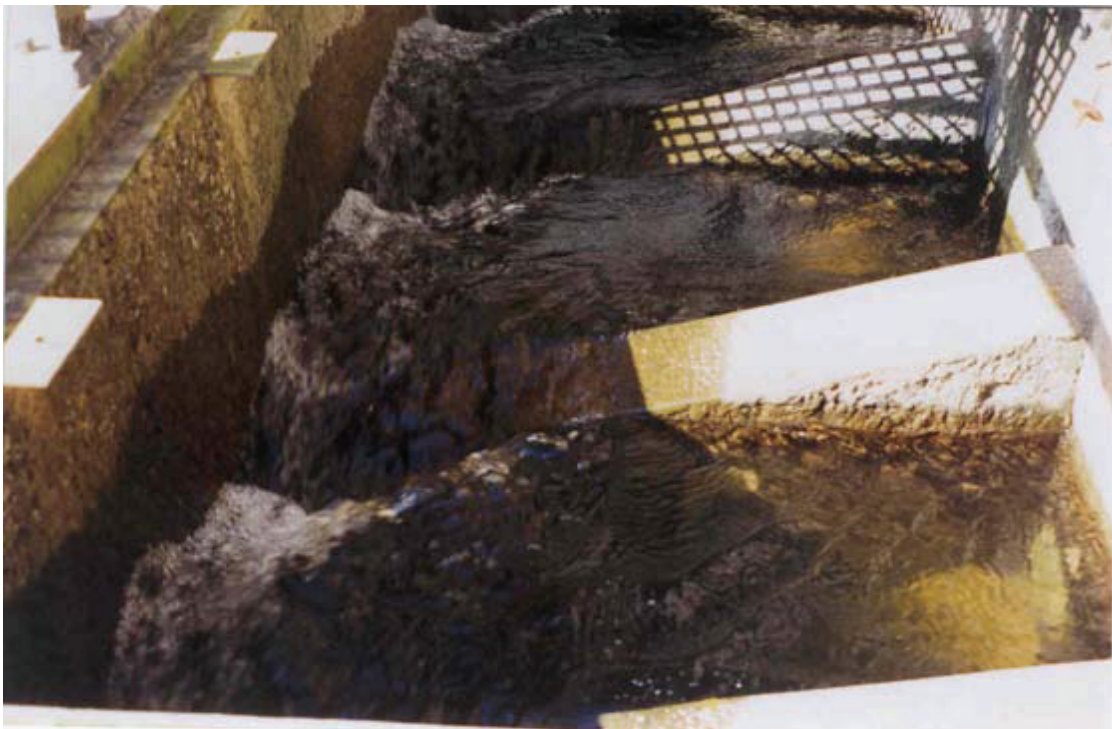
Figure 10-22 Close-up of sloping weir of the Nhlabane pool and weir fishway at low flows, looking up-stream (Bok et al.,2007)
