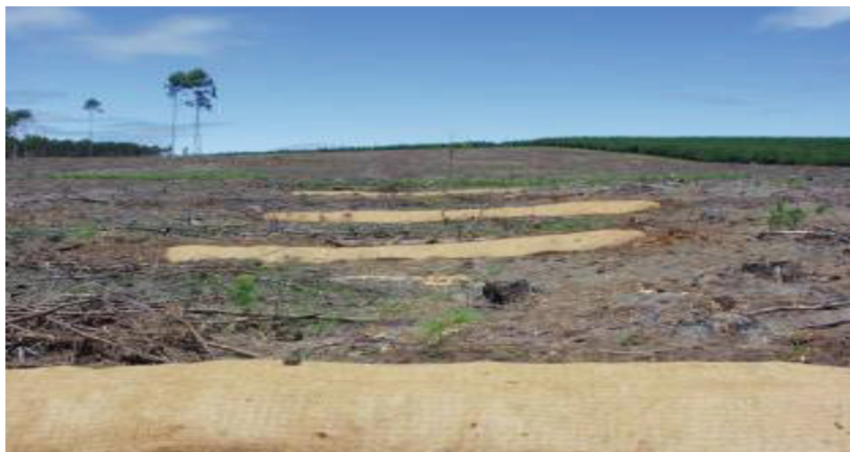
Figure 10-3 Fibre mats covering compacted soil berms in a seepage wetland that had previously been drained (Sieben et al. , 2007)
