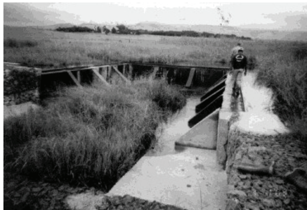
Figure 10-12 A U-shaped concrete buttress weir constructed on a gabion structure encased in concrete in a wetland environment (Russell, 2007)
