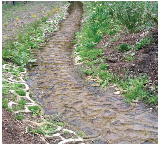
Figure 10-6 Terraforce blocks used for erosion protection of a channel bed (photo courtesy of Terraforce)
