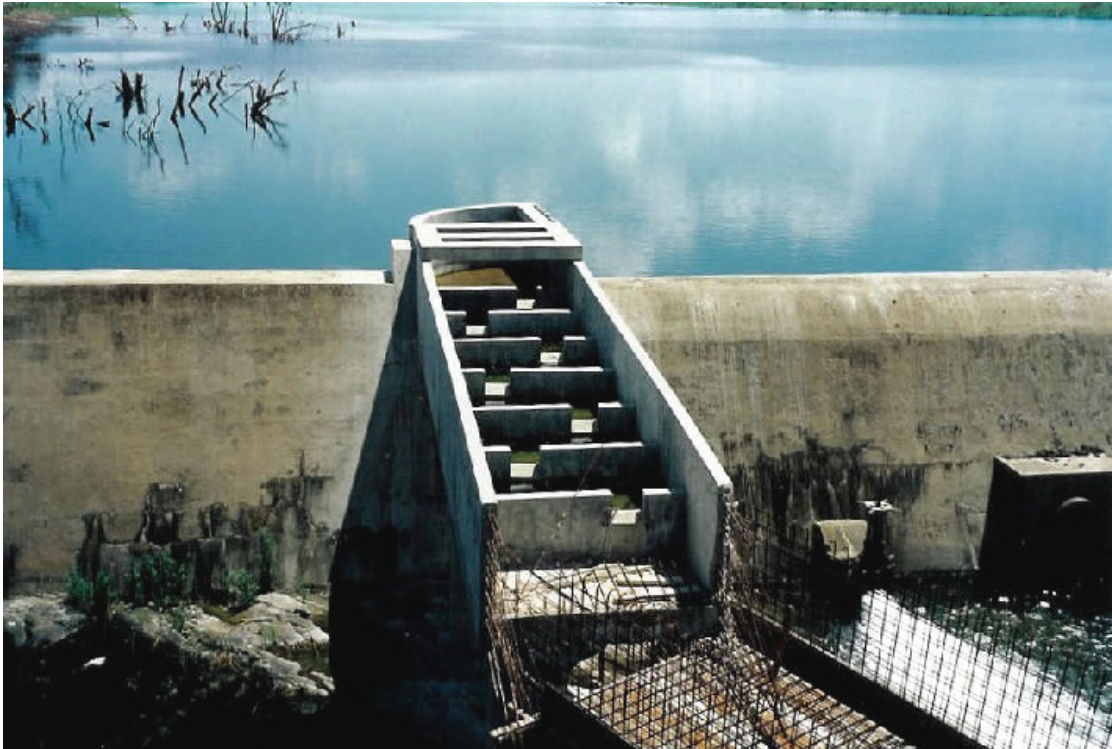
Figure 10-21 Pool and notched-weir fishway on the Lebombo gauging weir on the Komati River (Bok et al.,2007)
