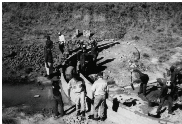
Figure 10-13 Building an arch weir, double walls of concrete bricks with concrete fill in-between. Planned for raising once the sediment has reached the spillway level (Russell, 2007)
