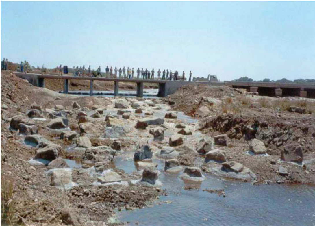
Figure 10-18 Bypass rockramp fishway on the Lower Sabie River in KNP under low flow conditions at commissioning in October 2001 showing placement of rocks (Bok et al. , 2007)
