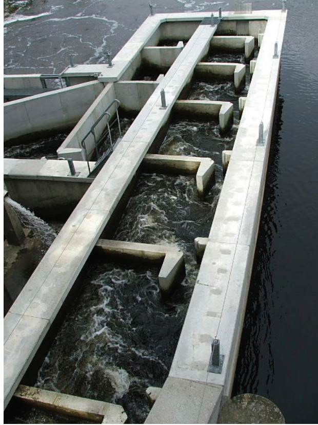
Figure 10-20 Large vertical slot fishway at Mauzak, France (Bok et al.,2007)
