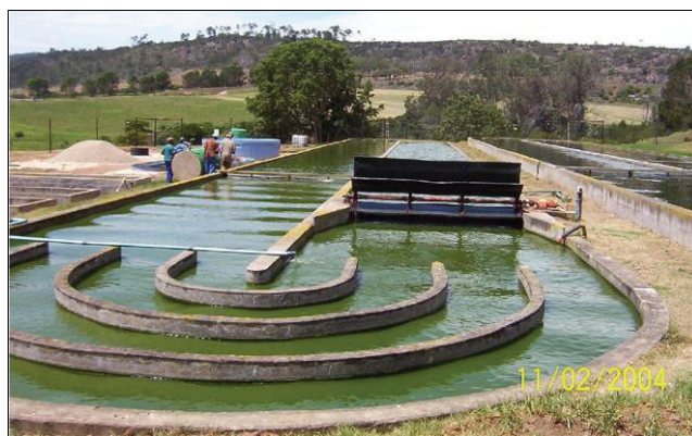
Figure 2.3: High-Rate Algal Ponds of the Integrated Algal Ponding System plant showing the paddle wheels and the flow path dividing walls.
