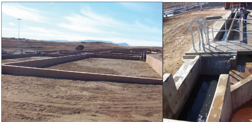
Figure A.20: The sludge drying beds at Mt. Frere activated sludge works (left) with the inlet works (right).
