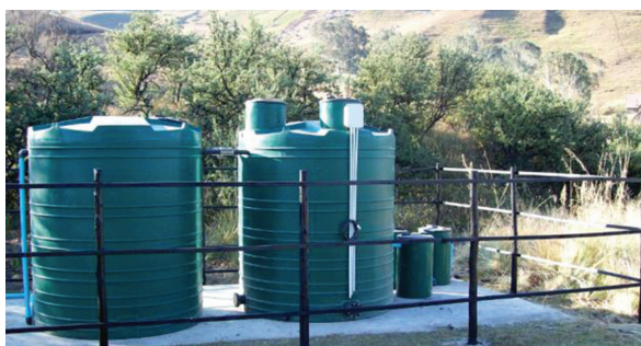
A typical small wastewater treatment system.
