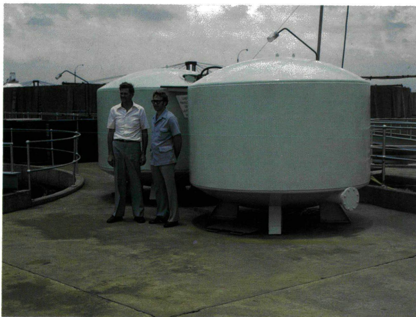
The works superintendent, Mr Henrie Basson (left) and the chief chemist, Mr Dries Louw, at the chemical storage tanks.
