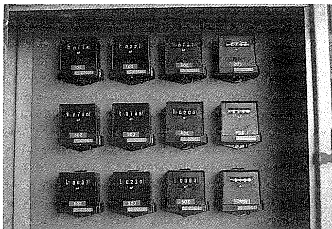
Remote registers of water meters installed at the individual units of Kiowa flats.
