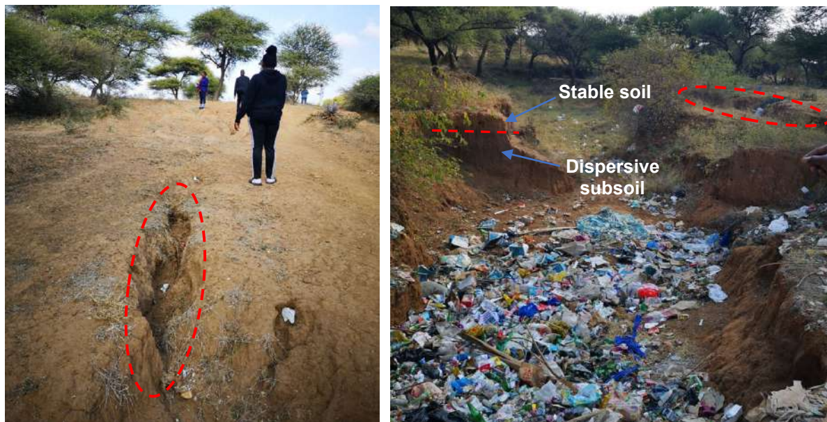
Figure 5.5 Development of gully erosion at Beauty (Mokolo); Left – bare land and steep slope contributing towards erosion, right – inherent soil erosion enhancing gully formation.
