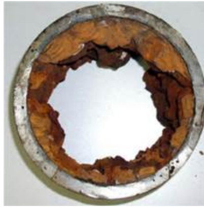
Figure 2.17: Cast iron rust tubercles ( http://dofbill.com/category/lead-poisoning/ )
