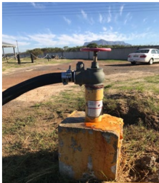
Figure 4.38: Installed fire hydrant head with the PCAE hosepipe connected
