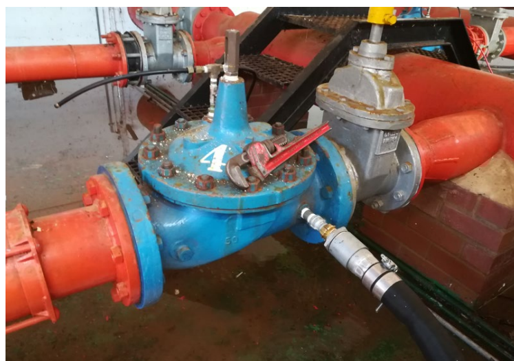
Figure 4.79: Connection point on the pressure-regulating valve
