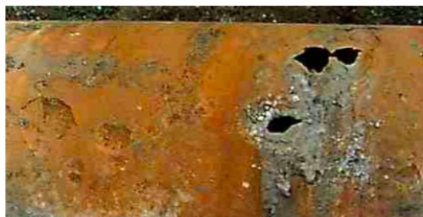
Figure 2.15: External corrosion of ductile iron pipes
