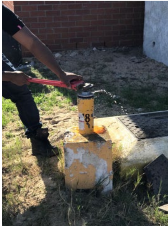
Figure 4.37: Covered fire hydrant
