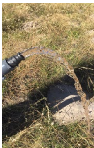
Figure 4.25: Clear water after flushing
