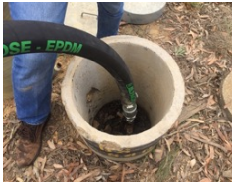
Figure 4.6: The PCAE hosepipe connected to the BS 8 pipeline
