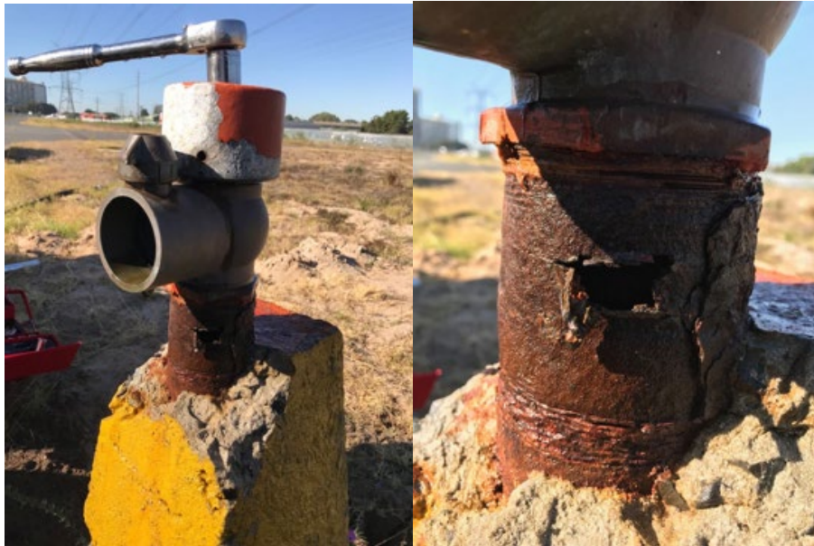
Figure 4.34: Failed fire hydrant pipe
