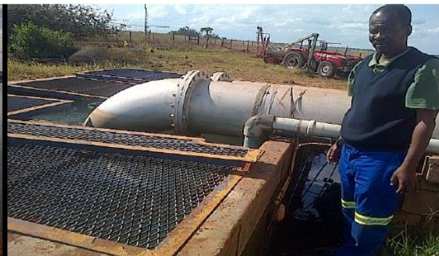
(b) The main irrigation pipe or canal
