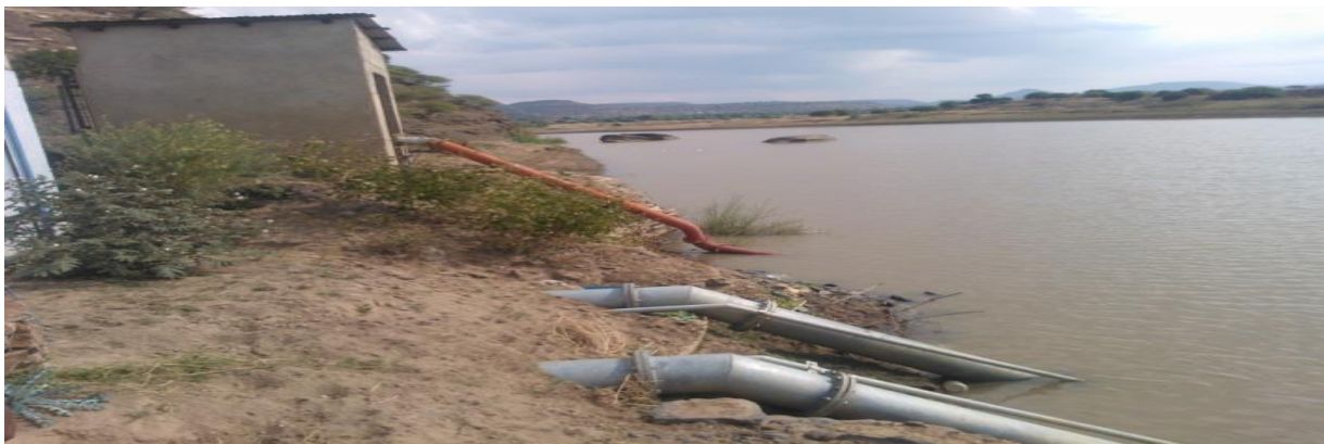
Figure 4.9. Pipes pumping water from the river to the dam
