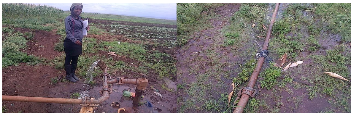
Figure 5.4. The status of pipes in Ndumo-B Irrigation Scheme
