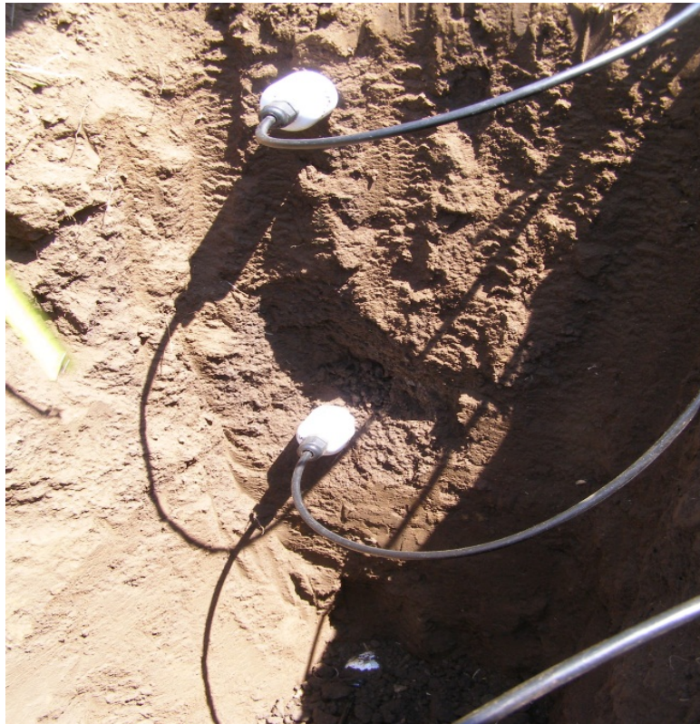
Figure 9. Three Hydra Probe II soil moisture sensors installed at 0.1, 0.5, and 1.0 m depths below the soil surface.
