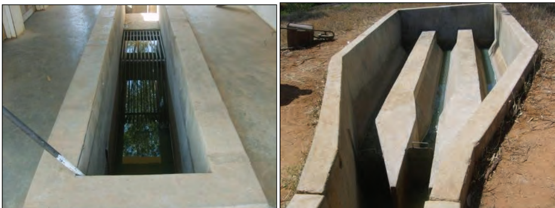
Figure B-1: Typical bar screen (left) and grit channels (right)
