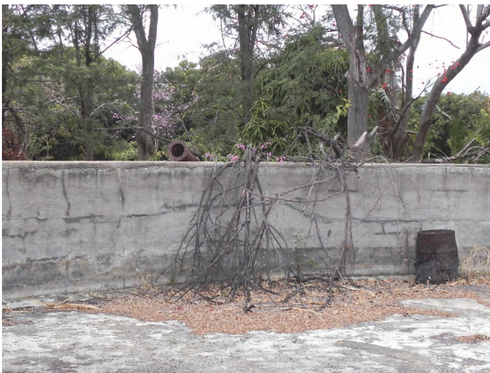
Photograph 6: A damaged disused reservoir on respondent D's farm
