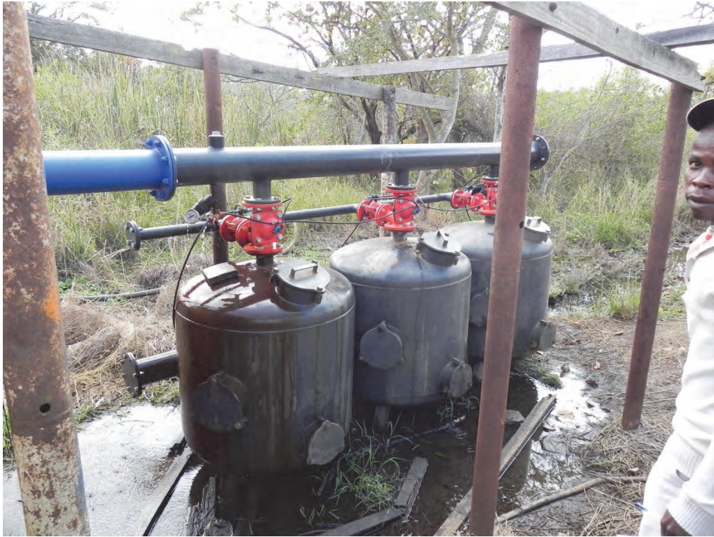
Photograph 21: Sand filter bank for pumping station of respondent G's farm
