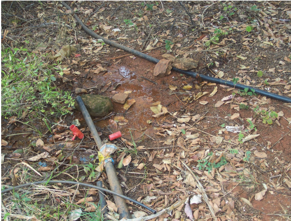
Photograph 5: Poor maintenance of irrigation system (respondent C)
