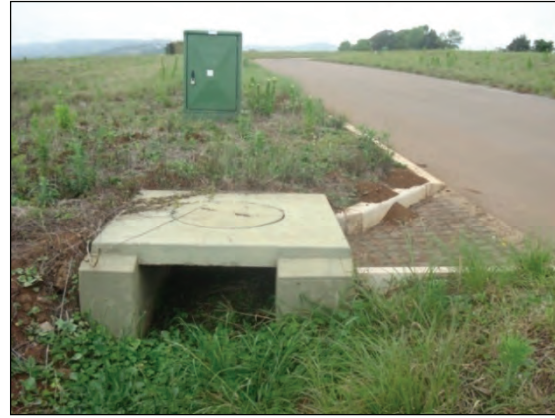
Figure 4-28: Road swale catchpit in Cotswold Downs
