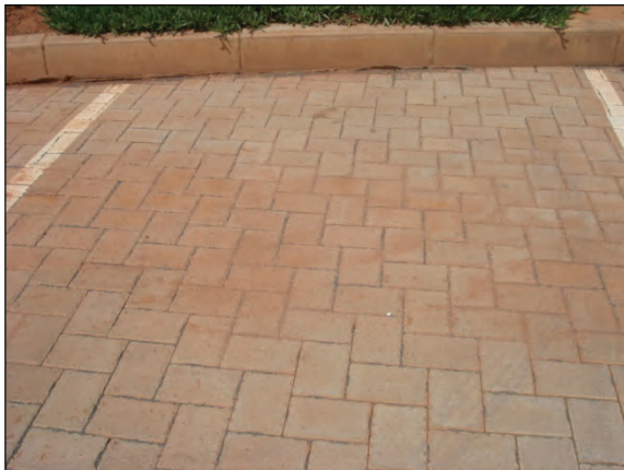
Figure 4-10: Sand and silt covering the permeable paving in the lower Wits parking area
