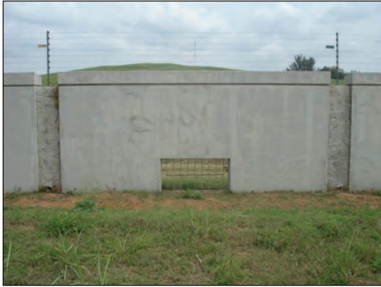
Figure 4-30: Rectangular drainage opening in the boundary wall at Hawaan Estate
