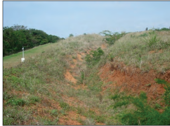
Figure 4-35: Large connecting infiltration trench in Hawaan Estate
