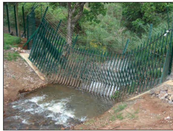
Figure 4-26: Large trash rack on the Nkutu River
