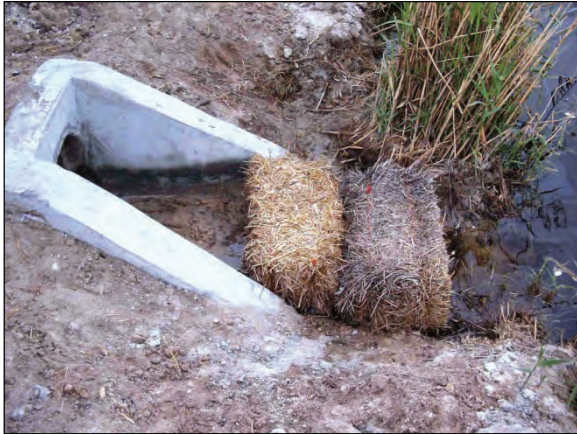
Figure 4-43: Barley straw bales at canal network inlet in Century City
