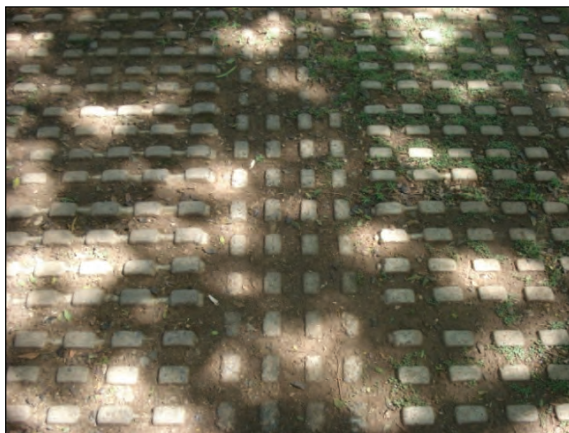
Figure 4-13: Unattractive concrete grass block paving with dead grass
