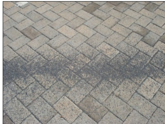
Figure 4-11: Stone fines and crusher dust covering the permeable paving in the Wits parking area
