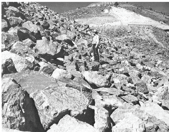
Figure 9.1-2 Example of relatively large rock grading as riprap protection on the upstream face of an embankment dam wall (USBR, 1987)
