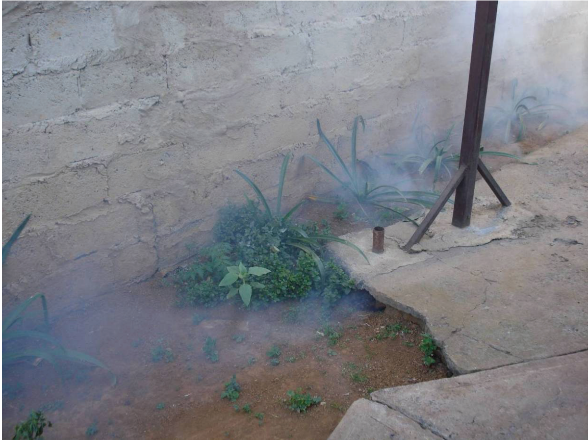
Figure A3: Smoke pours out of the ground revealing the location of a broken section of domestic sewer. In this case the home owner may not be aware of the problem with the sewer pipe, but such a section of pipe will function as a subsoil drain, carrying away stormwater when it rains. This kind of sewer break would be hard to find using a routine visual inspection of the yard.
