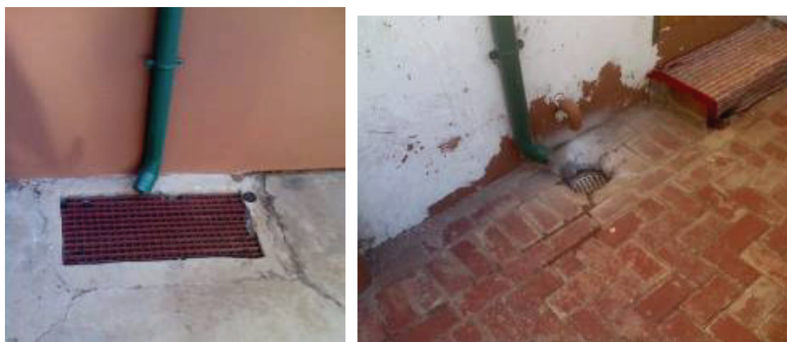
Figure 5: Roof gutters directed into sewer lines (Source: Pienaar, 2007)
