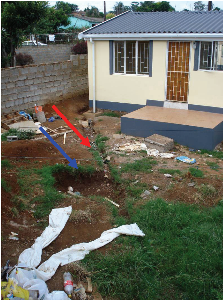
Figure 25: The red arrow shows a trench designed to route stormwater to the sewer (off camera), while the blue arrow shows what appears to be intended as an inline soakpit.
