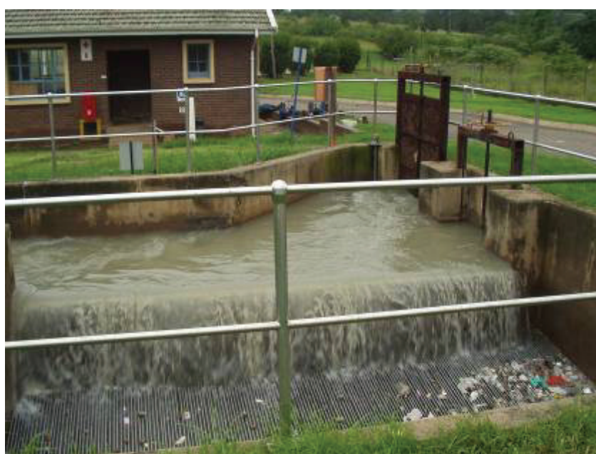
Figure 7: Darvill WWTW overflowing to the storm dam during a routine wet weather event
