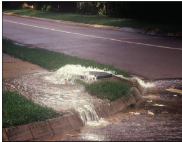
Figure 1: Wastewater overflowing (not held under pressure)
