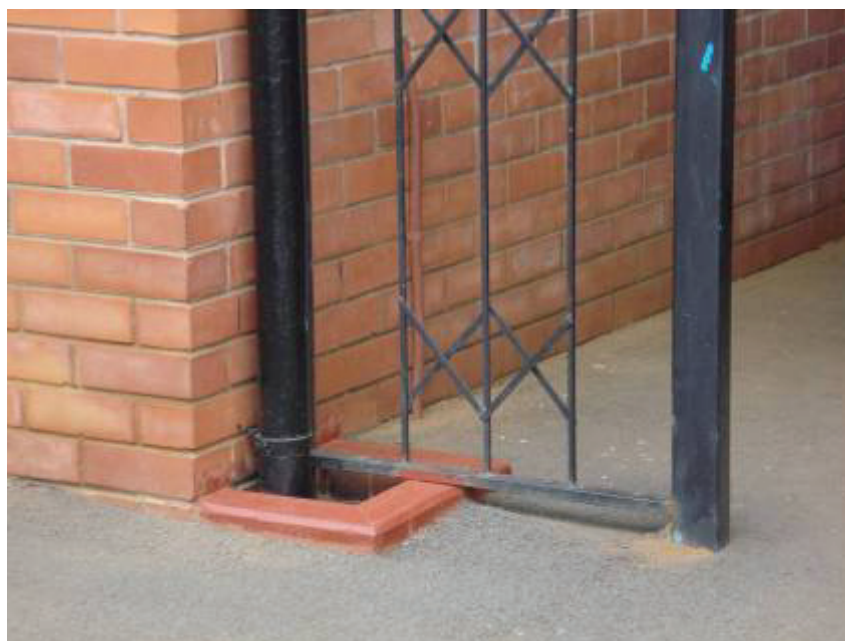
Figure 24: A downpipe from a home in Lotusville disappearing into a gully – where does the water go?
