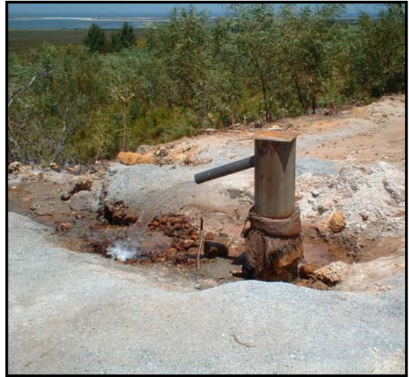
Uncontrolled discharge from artesian boreholes could result in erosion. Measures must be put in place to avoid such impacts.
