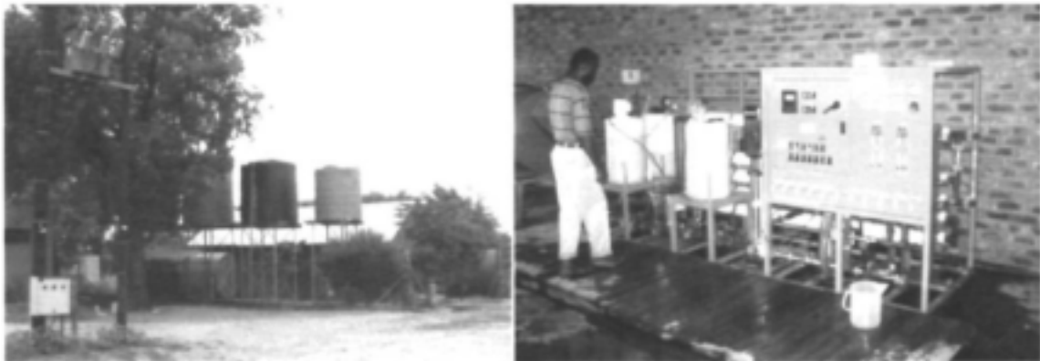
Figure 18: Desalination plant at nZava with power supply and storage tanks (left) and deionization unit (right) with operator
