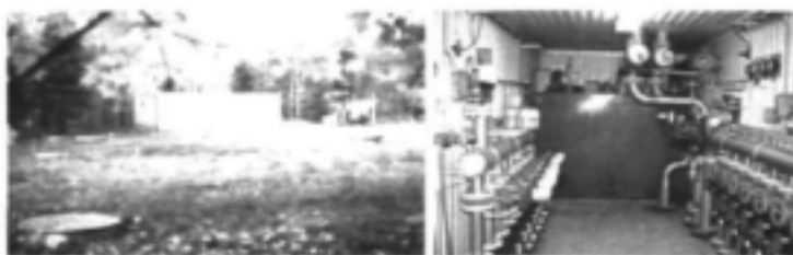
Figure B3 Control room location and pipework (right)
