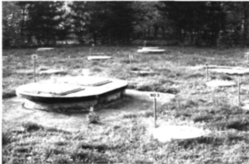
Figure 20: Bisamberg in situ denitrification system, with abstraction well (EB) on the left
