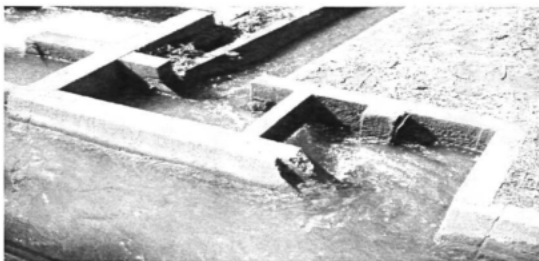
Photo 5.4 Vandalism of irrigation delivery structures like a canal sluice gate at Tshiombo irrigation scheme prevent effective water distribution on the scheme (2003)
