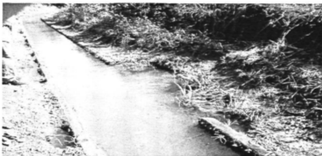
Photo 5.3 Poor maintenance of secondary irrigation canals and excessive vegetative growth on the canal banks at Tshiombo irrigation scheme (irrigation blocks 3 & 4) often cause inefficient water distribution efficiency.
