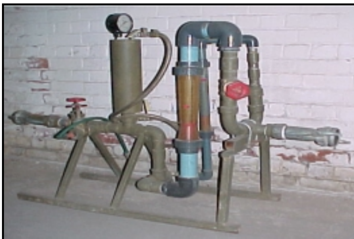
Fig. A11 Flow meter to measure discharge from pump
