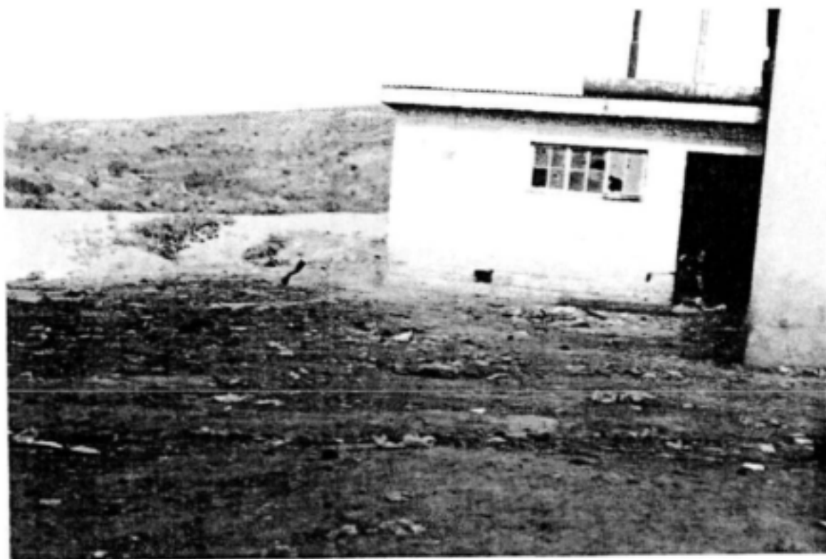
Photo 2: Defecation at Open Places at Tipini
