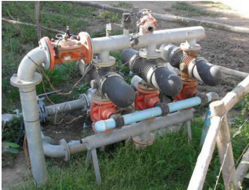
Fig. 5.2 Existing disc filtration system on the farm.
