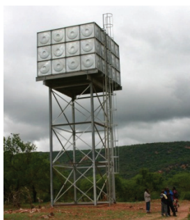
Figure 2.6b: Clean-water holding tank
