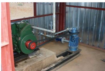
Figure 2.5a: Motorised pump on borehole
