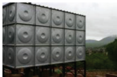
Figure 2.5b: Clean-water holding tank
