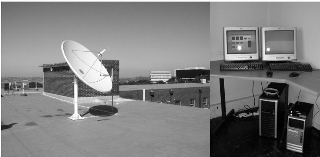
Figure 3.4 The Meteosat-8 receiving station at UKZN. The left-hand panel shows the installed antenna on the roof of the Durban Centenary Building. The right-hand panel shows the receiving PC and Data Server.
