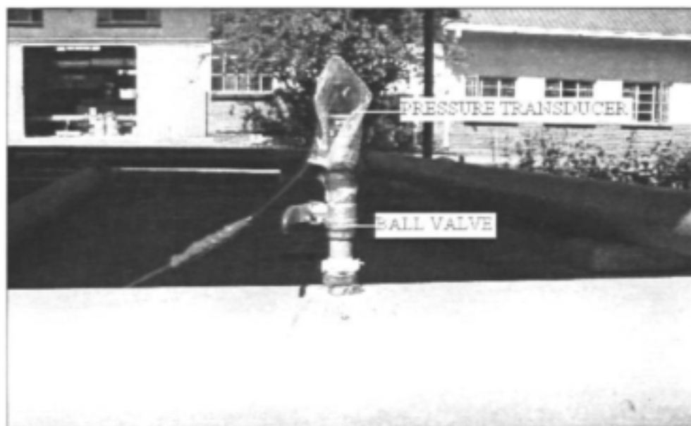
Figure 4.4.7: Pressure transducer at the upstream end of the leakage
