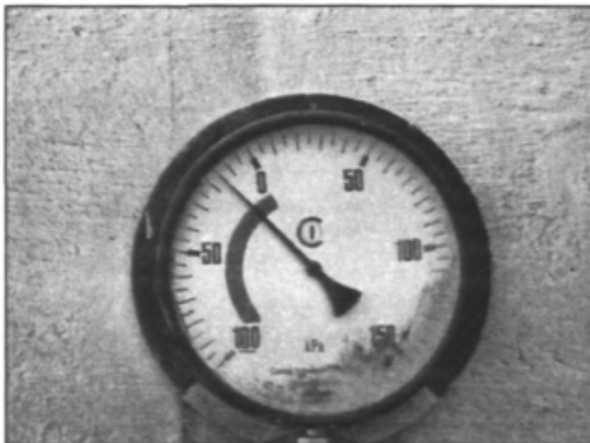
Figure 3.4.4: Negative pressure on the suction side of the pumps
