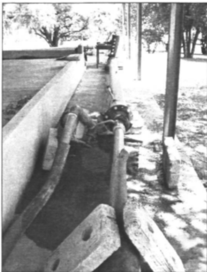
Figure 4.4.12: View of system layout looking upstream from the ball valve at the end of the pipe
