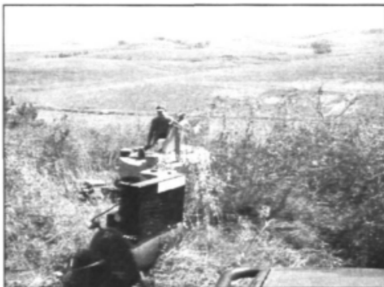
Figure 3.2.5: Air induction facility (compressor)
