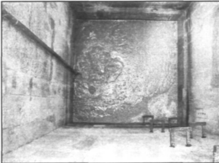
Figure 3.4.2: Fizzing water in the surge tower
