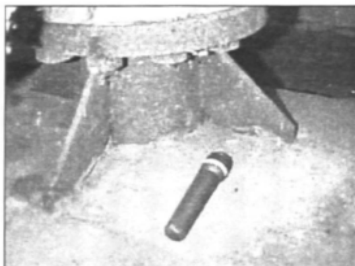
Figure vii: Typical 100 mm off-take (stub) underneath the air valve
