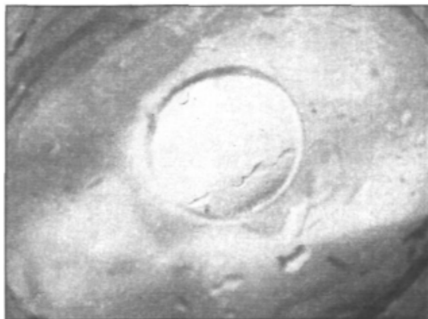
Figure 4.3.11: The discontinuity of 30% of the diameter in the pipeline
