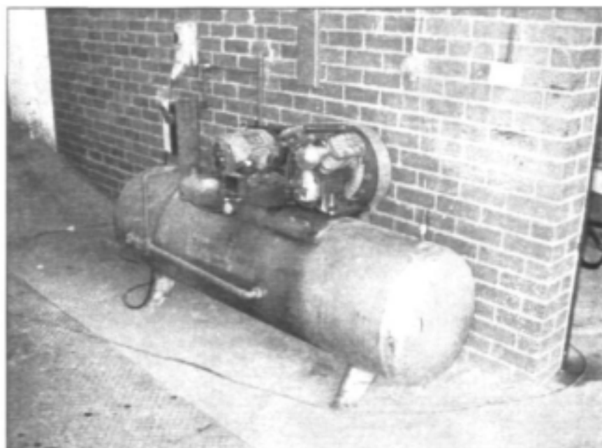
Figure 4.2.7: The compressor used for supplying air
