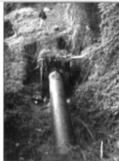
Plate 23.3 (Locality not exact). Showing erosion and alien encroachment around sewerage pipeline at top of left bank
