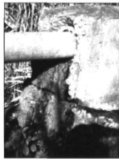
Plate 18.3 Close-up of slow, constant leak in sewage pipebridge, where raw sewage trickles into the river.
