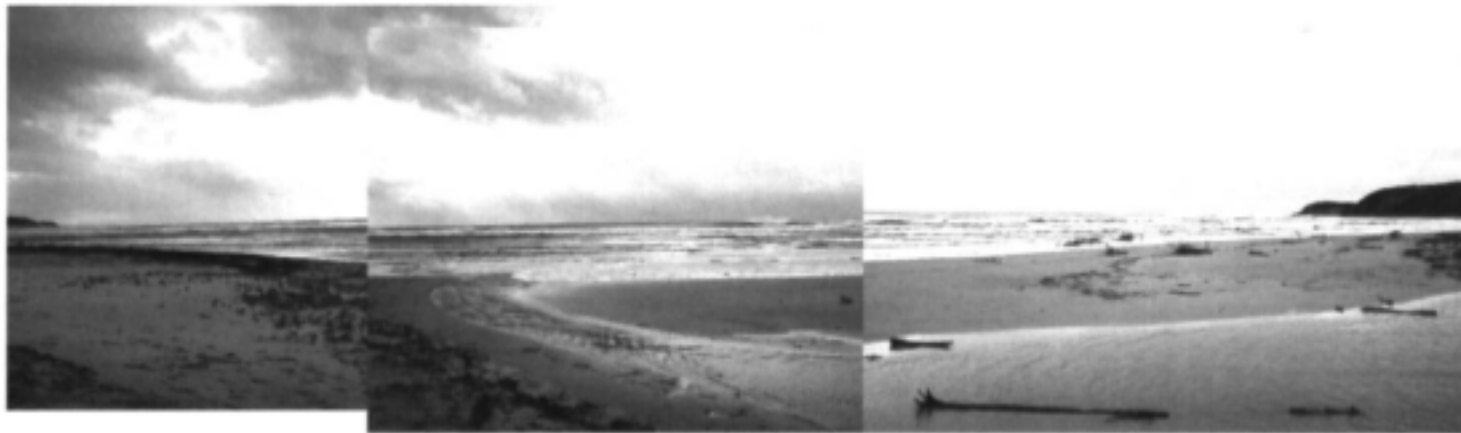
Plate 30.2 The sewage pipe bridge across the estuary in Reach 20. This pipe continues up over the dune system visible in Plate 30.1 and leads to Hood Point Sewerage Treatment Works.
