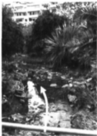
Plate 5.1 Channel at top of Reach 5
