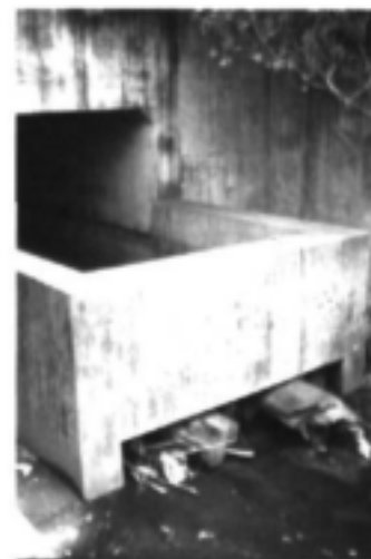
Plate 10.2 Blockage in the stilling well
