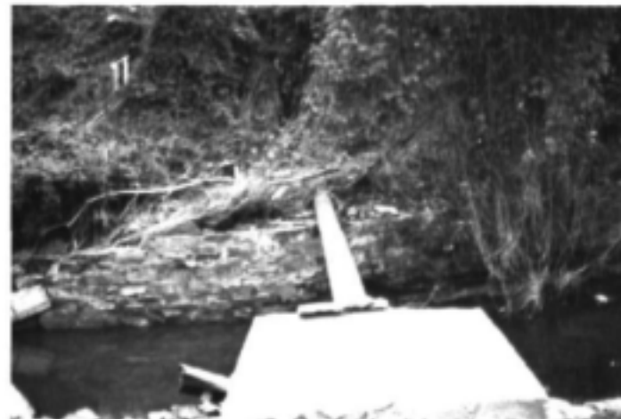
Plate 3.1 Sewage pipe bridge across upper section of the channel in Reach 3, immediately downstream of Chamberlain Rd bridge.
